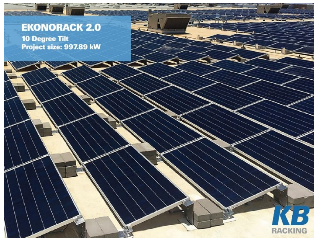
Figure 3-9: An example of a KB Racking EkonoRack 2.0, 1MW, 10 degree tilt installation
