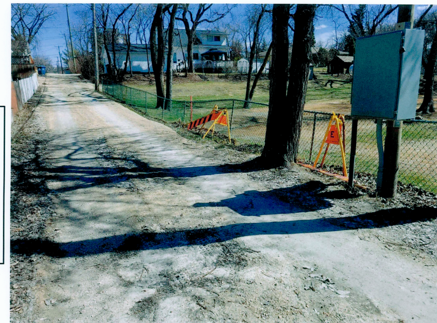
IRVING PLACE BACK LANE TEMPORARY PUMP STATION
