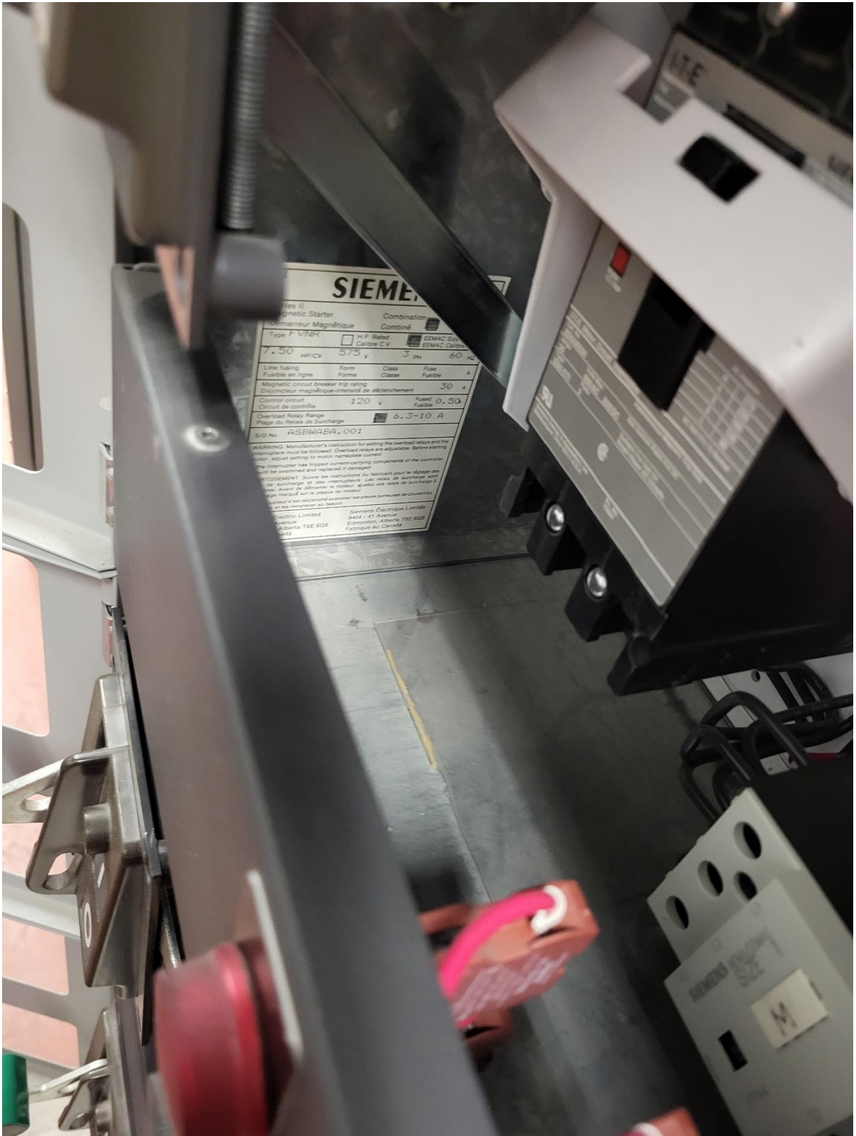
Figure 11: Existing MCC bucket information.
