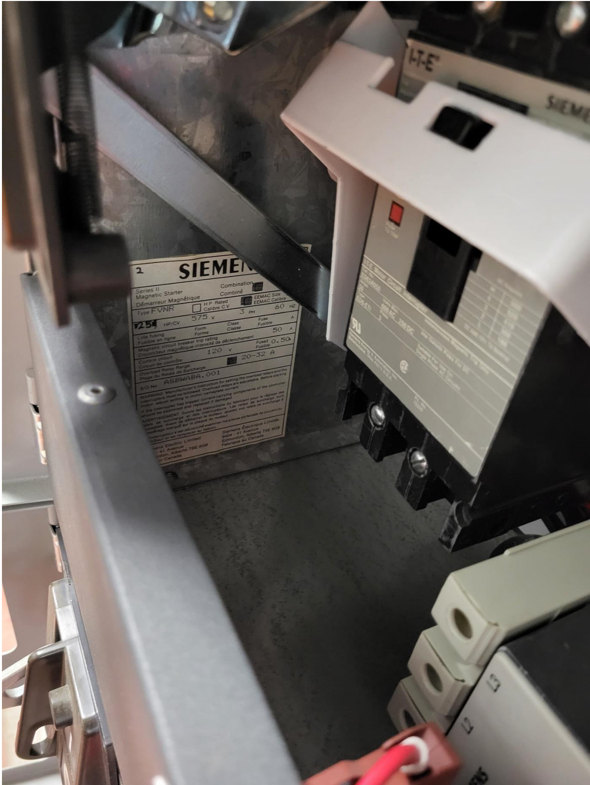
Figure 5: Existing MCC bucket information.
