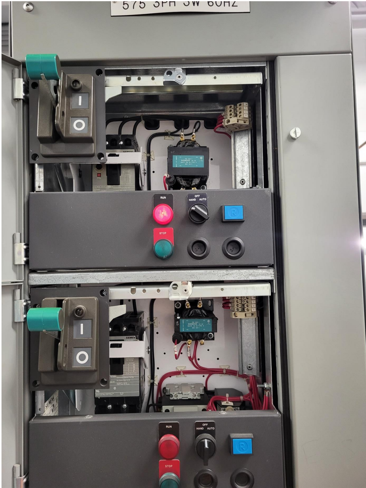
Figure 15: Existing MCC bucket.
