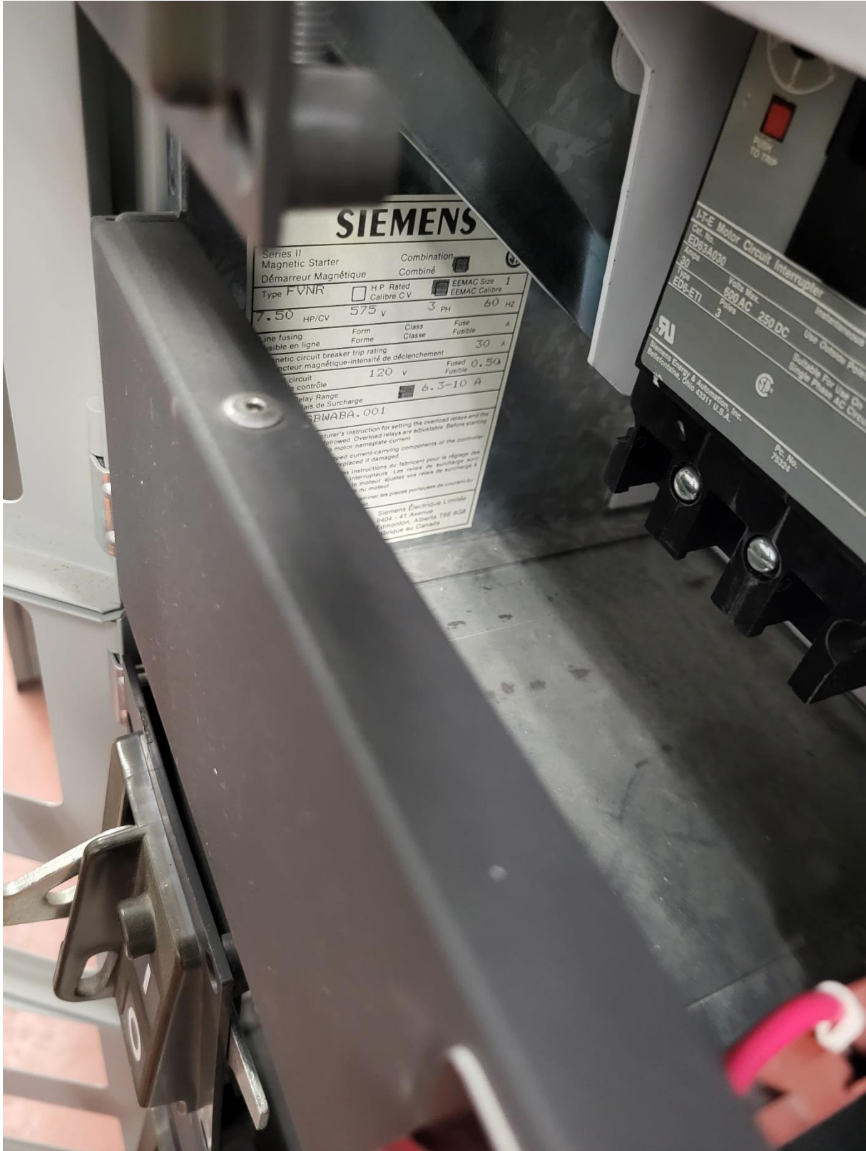
Figure 8: Existing MCC bucket information.
