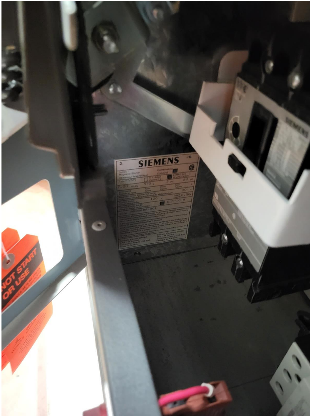
Figure 3: Existing MCC bucket information.
