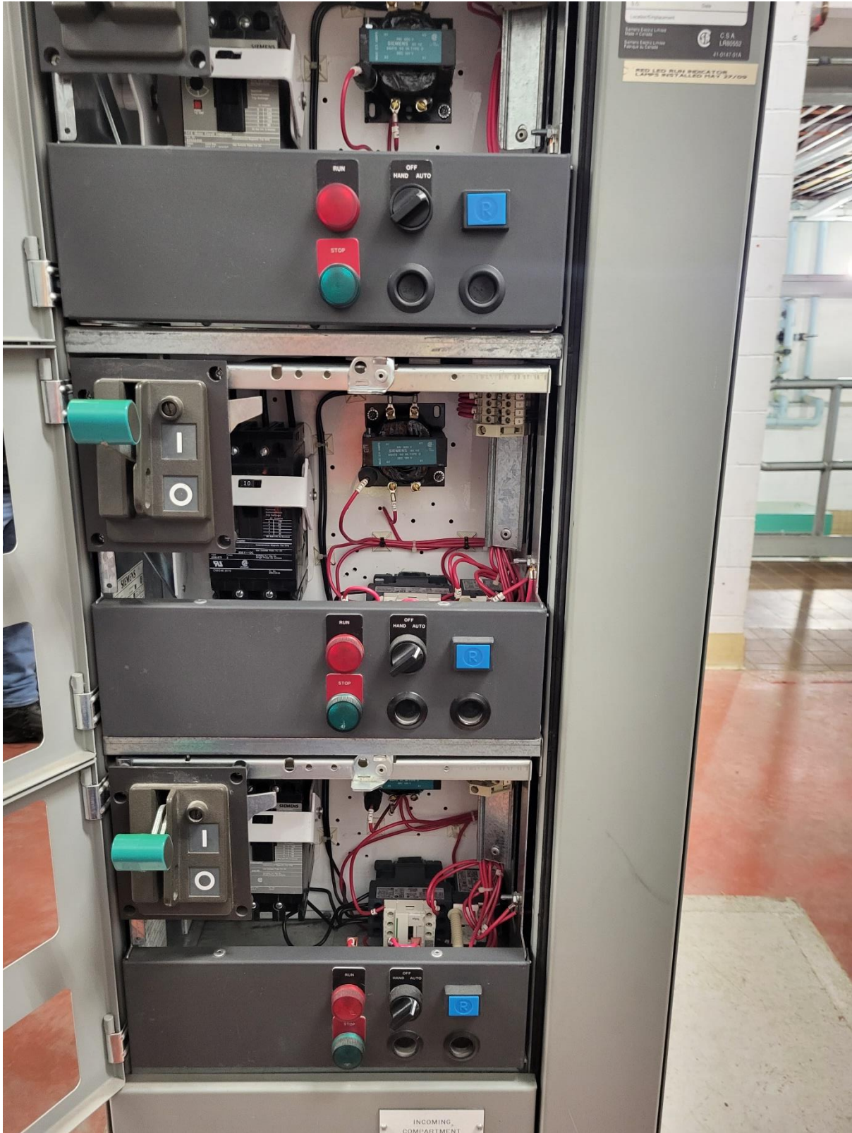
Figure 13: Existing MCC bucket.
