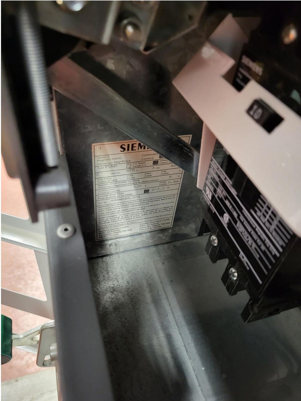
Figure 9: Existing MCC bucket information.
