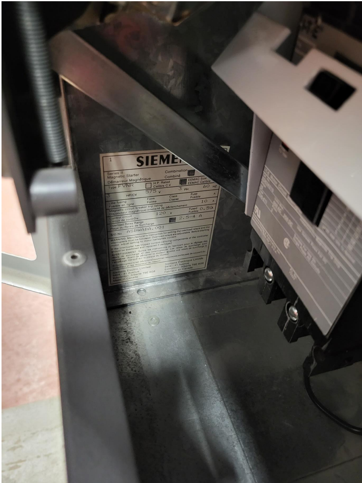
Figure 10: Existing MCC bucket information.
