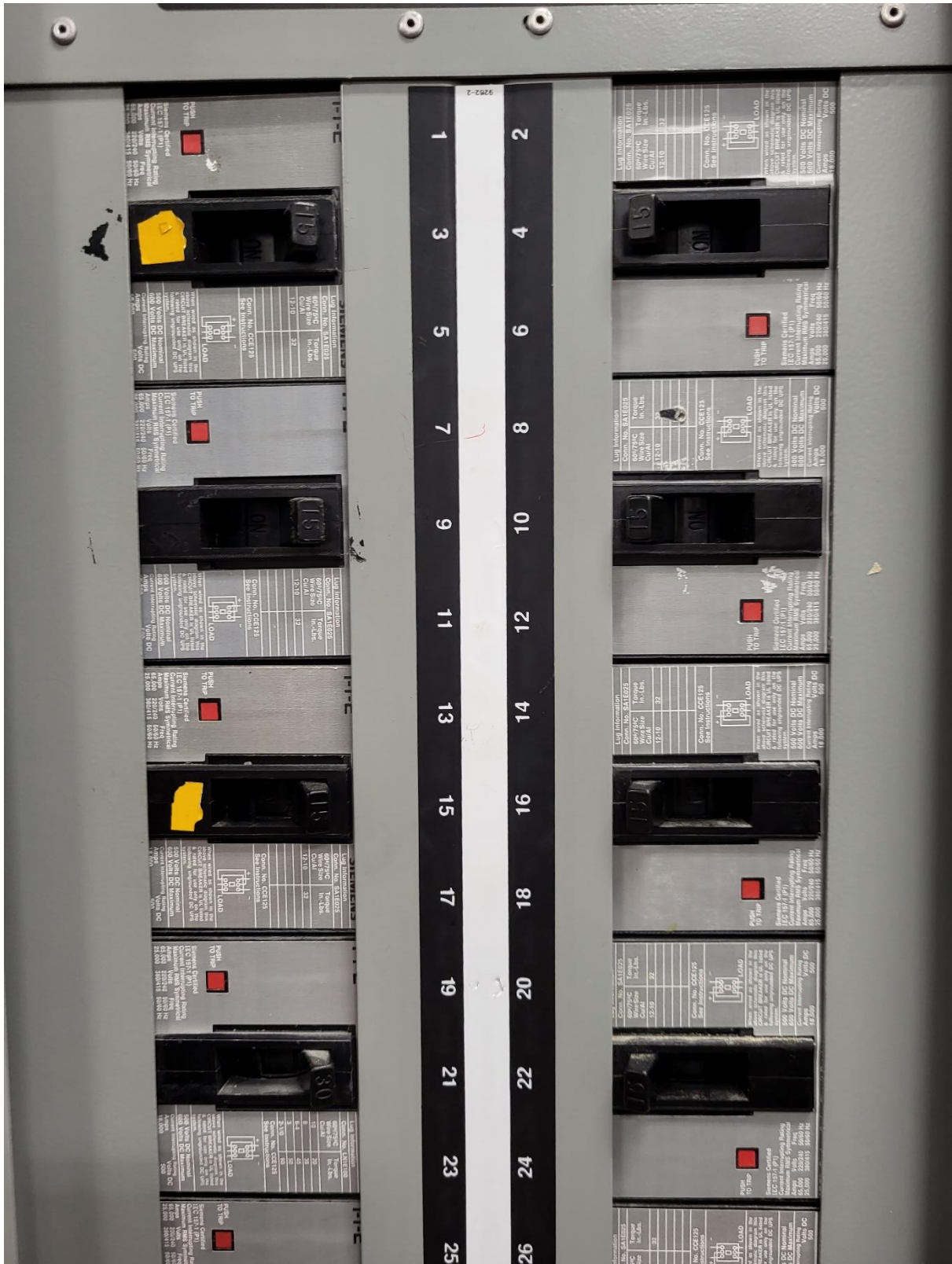
Figure 2: Existing Panel EE photo #2.
