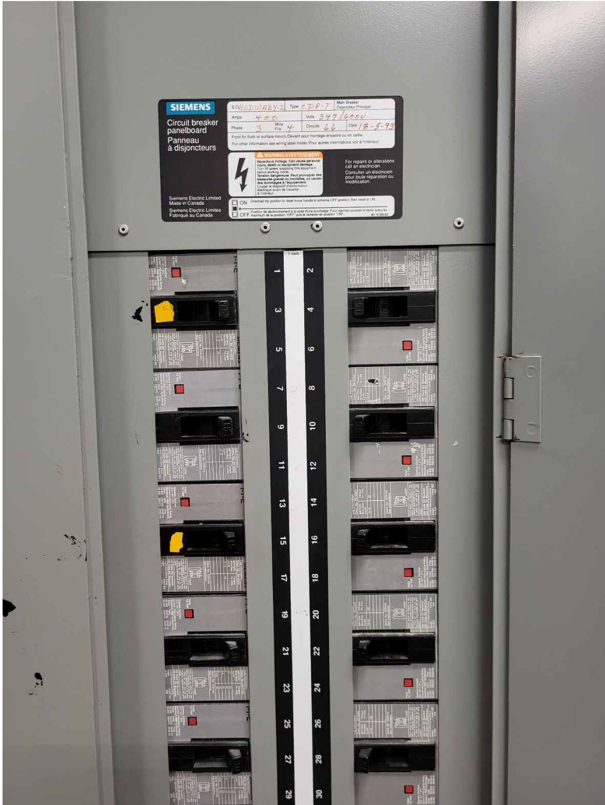
Figure 1: Existing Panel EE photo #1.
