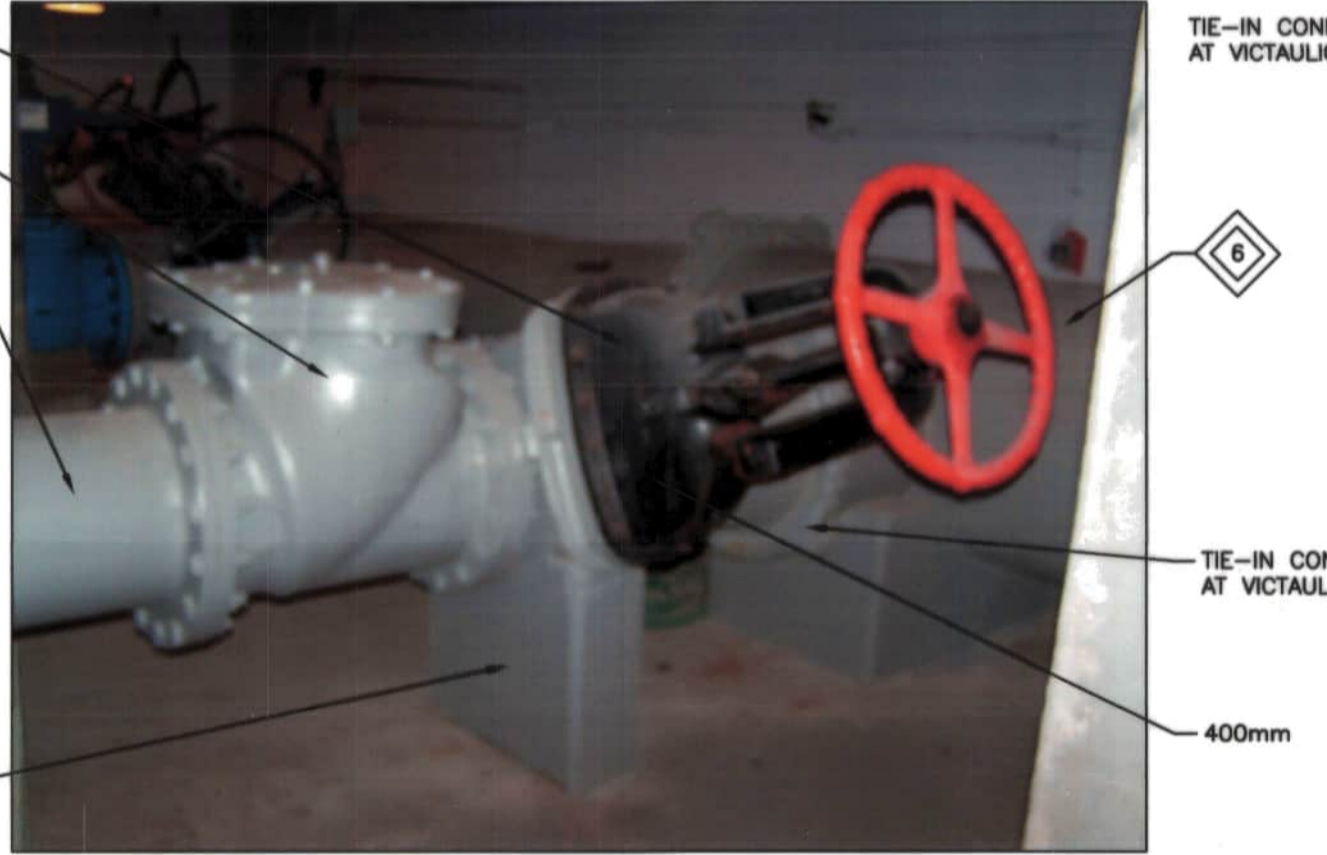
7 P3 DISCHARGE PIPING - LEVEL 200 M1
