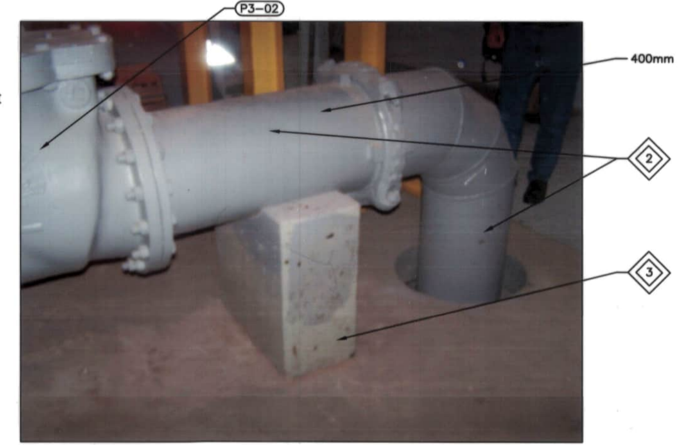
6 P3 DISCHARGE PIPING - LEVEL 200 M1
