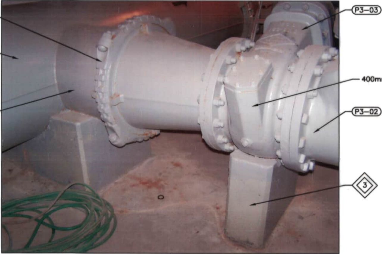
8 P3 DISCHARGE PIPING - LEVEL 200 M1
