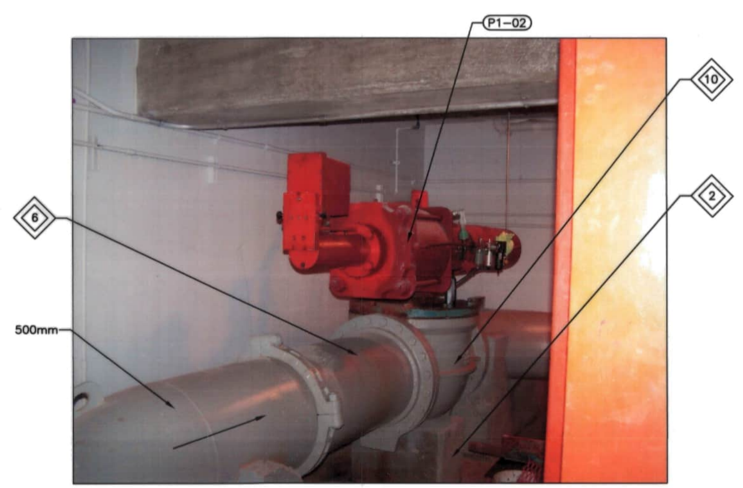
8 SHUTDOWN 7 - CONTROL VALVE P1-02 M2
