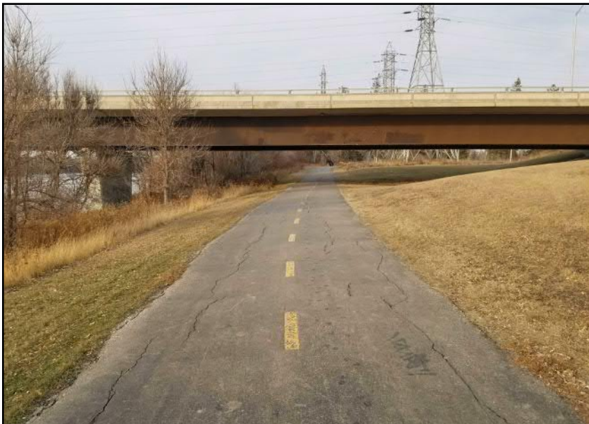
Site 4 - Eastern Riverbank Asphalt paved pedestrian pathway. Minor cracking observed parallel to bank crest (facing N)
