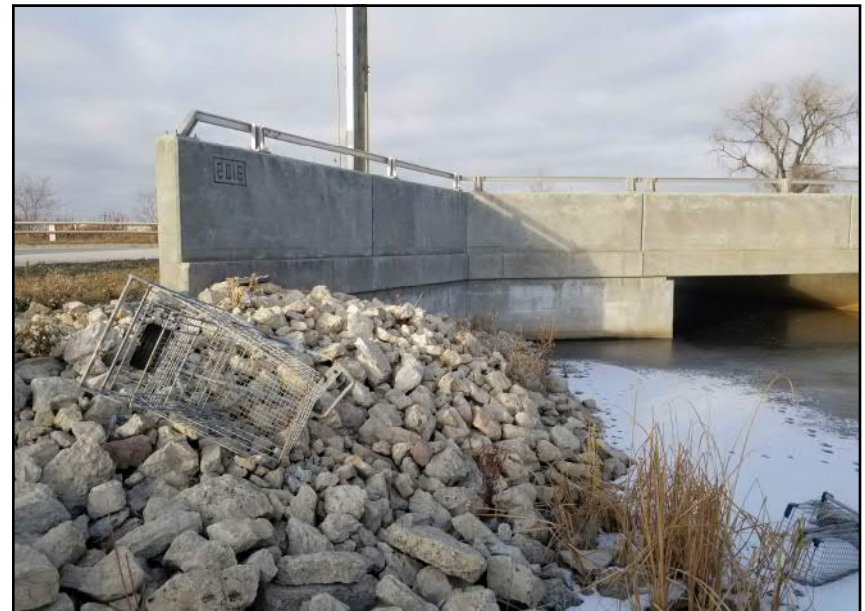
Site 8 - Western Bank | Regraded and rip-rap armoured slope near bridge structure. Steeper slope near abutment (facing N)
