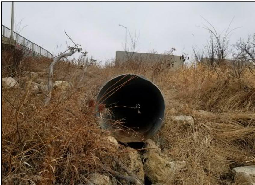
Site 5 - Northern Riverbank CSP outfall daylighting along bank slope, some erosion of bank material between rip-rap (facing N)
