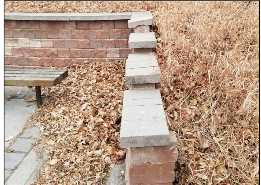
Site 10 - Northern Riverbank Masonry retaining wall structure near pedestrian pathway shows small signs of movement (facing W)
