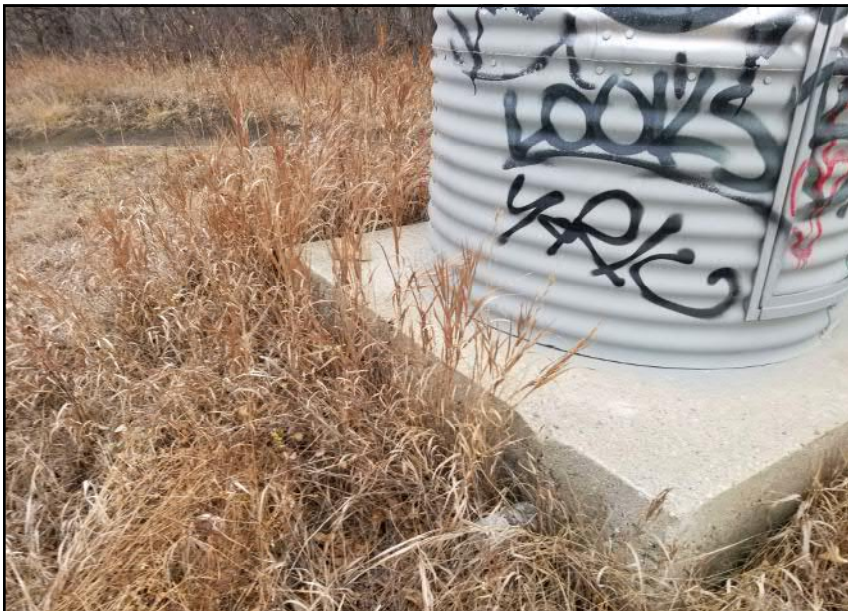
Site 5 - Southern Riverbank | No observed movement of lift station located at east crest of rip-rap drainage channel (facing E)
