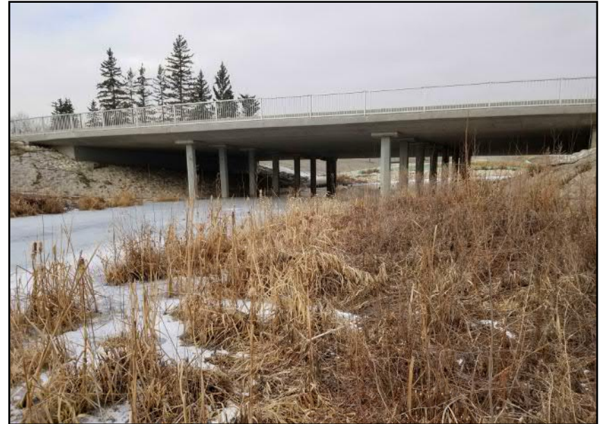
Site 7 - Eastern Bank Bank toe within southern portion of study area, indicating higher than usual water level (facing NW)
