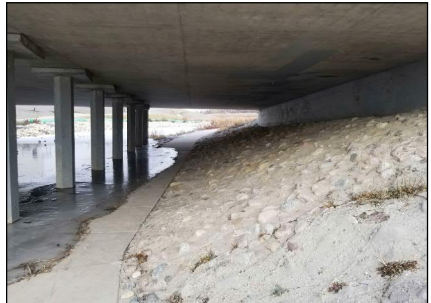
Site 7 - Eastern Bank Grouted rip-rap along abutment head slope below bridge structure (facing N)
