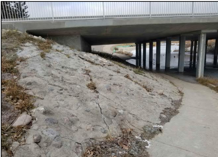
Site 7 - Western Bank Grouted rip-rap armorment along steeper banks in close proximity to bridge abutment (facing N)
