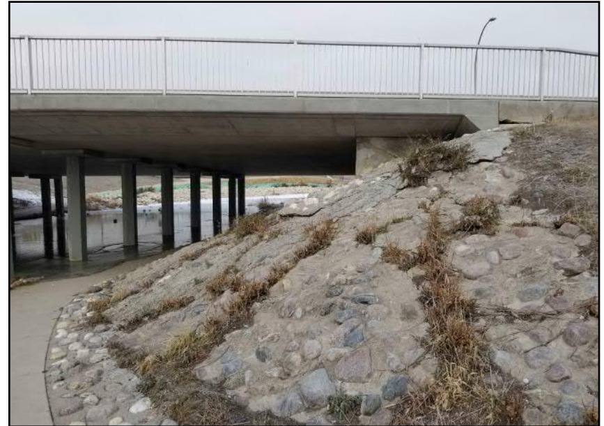
Site 7 - Eastern Bank Grouted rip-rap armouring along steeper banks in close proximity to bridge abutment (facing N)
