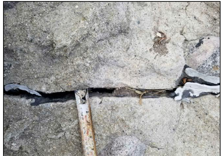
Site 7 - Western Bank Cracks observed within grouted rip-rap armorment at various orientations
