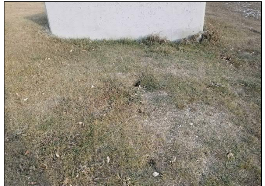
Site 4 - Eastern Riverbank Animal burrows observed in front of siphons inlet chamber structure (facing W)
