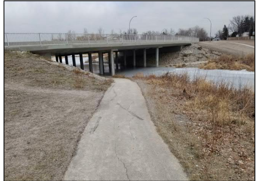
Site 7 - Western Bank Steeper slope around bridge abutment and minor cracking along pedestrian pathway (facing NE)
