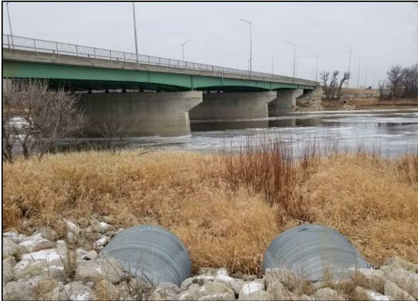
Site 5 - Southern Riverbank Discharge path of CSP culverts west of crossing alignment, gradual bank slopes (facing NW)
