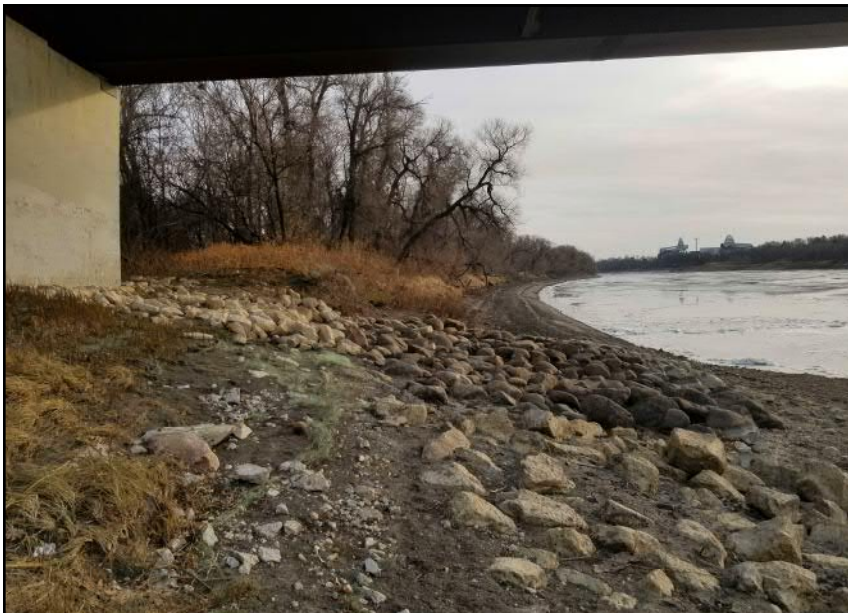
Site 4 - Eastern Riverbank | Rip-rap armoring around south bridge pier and along gradually sloping bank toe (facing S)
