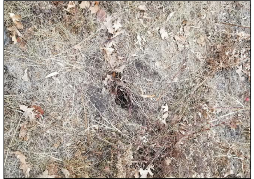
Site 9 - Western Bank Animal burrows observed within bank slopes.
