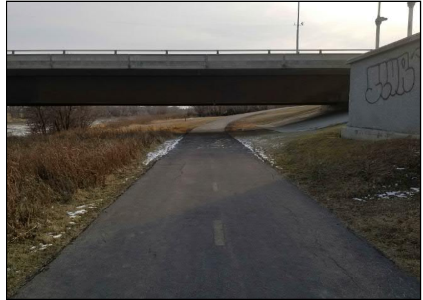
Site 4 - Western Riverbank | Asphalt paved pedestrian pathway. Minor cracking observed parallel to bank crest (facing S)
