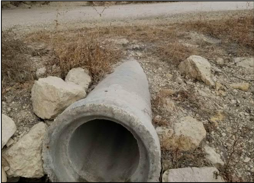
Site 5 - Northern Riverbank Concrete drainage culvert beneath roadway near bank crest close to bridge structure (facing N)
