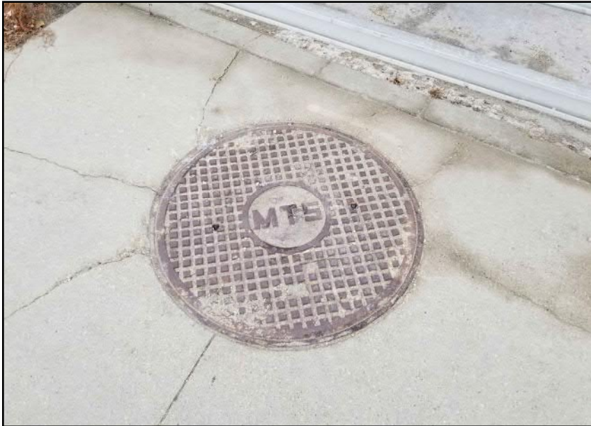
Site 7 - Western Bank Cracks around MTS manhole located in paved bridge sidewalk near abutment
