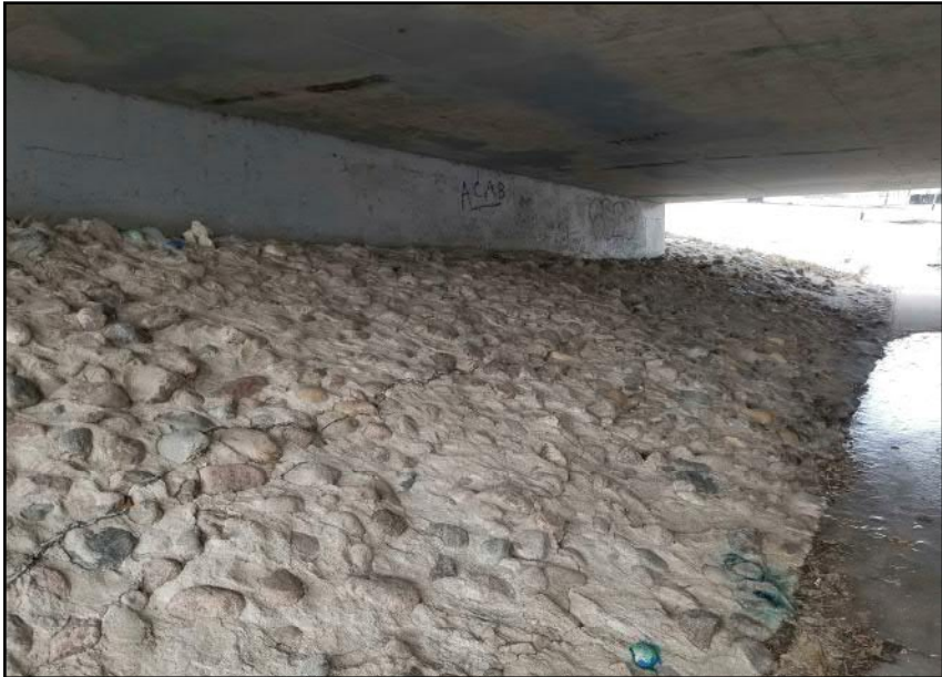
Site 7 - Western Bank Grouted rip-rap along abutment head slope below bridge structure (facing NW)
