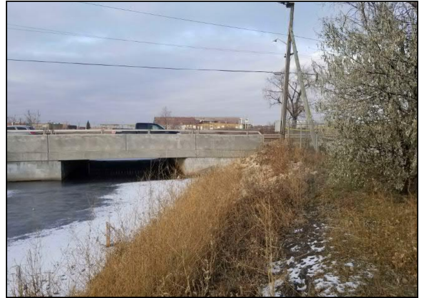
Site 8 - Eastern Bank Observed bank slope change due to regrading near start of rip-rap area (facing N)
