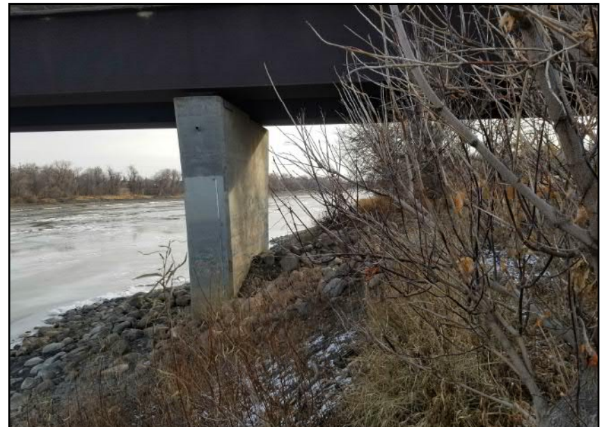
Site 4 - Western Riverbank | South bridge pier near river edge surrounded in rip-rap armouring (facing S)
