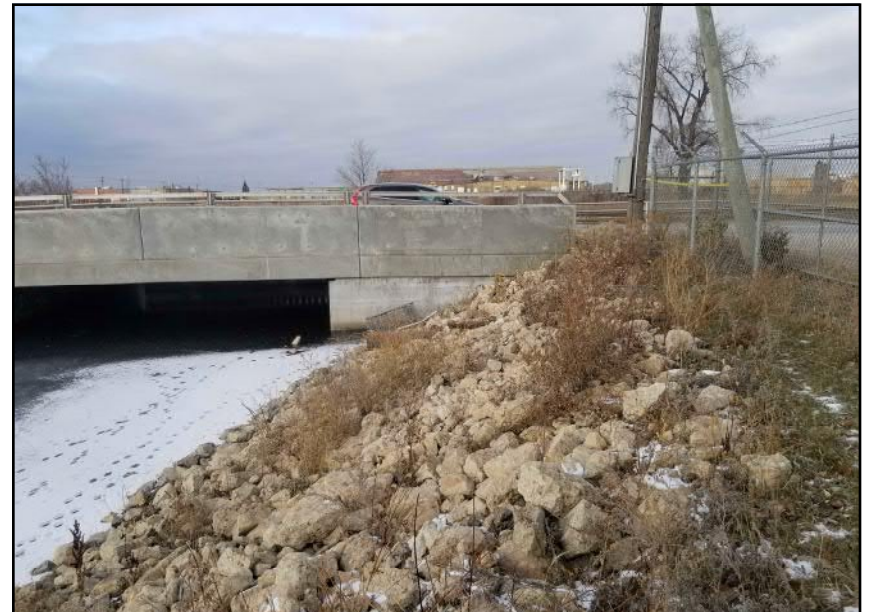
Site 8 - Eastern Bank | Regraded and rip-rap armored slope near bridge structure (facing N)
