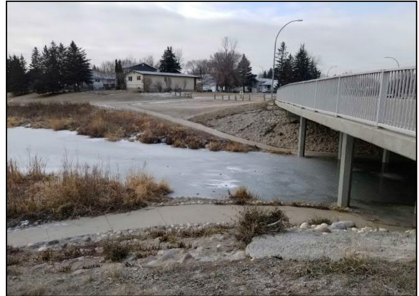
Site 7 - Eastern Bank | Steeper bank slopes close to bridge structure, under-bridge pedestrian pathway (facing W)
