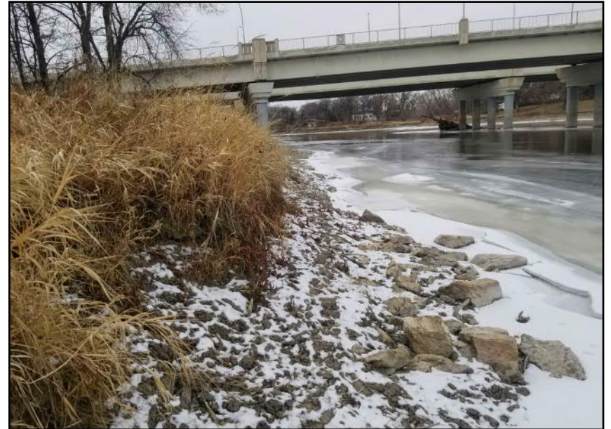
Site 10 - Southern Riverbank Local rip-rap observed along the bank toe near the crossing alignment (facing W)
