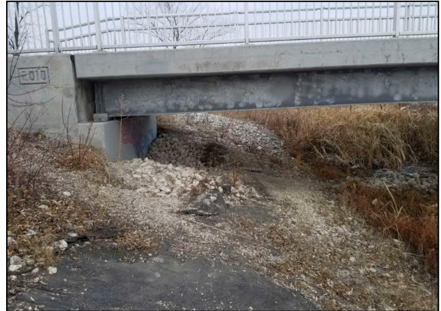
Site 9 - Western Bank Displaced rip-rap and exposed geotextile at bridge abutment north of the crossing (facing NW)
