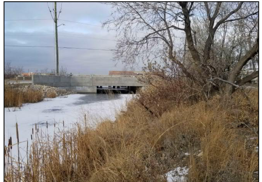
Site 8 - Eastern Bank Oversteepened banks observed within southern portion of the study area (facing N)
