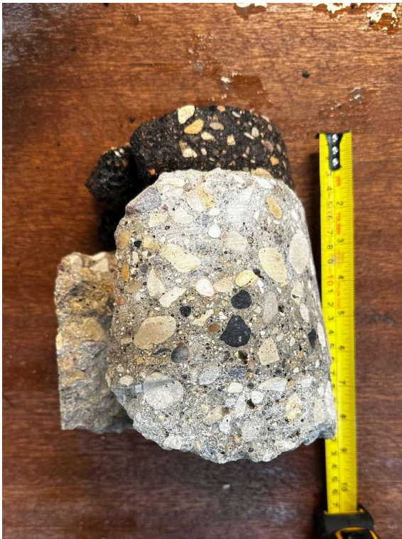
Figure 1. Core 1 pavement surface showing void existed between pavement and subsurface
