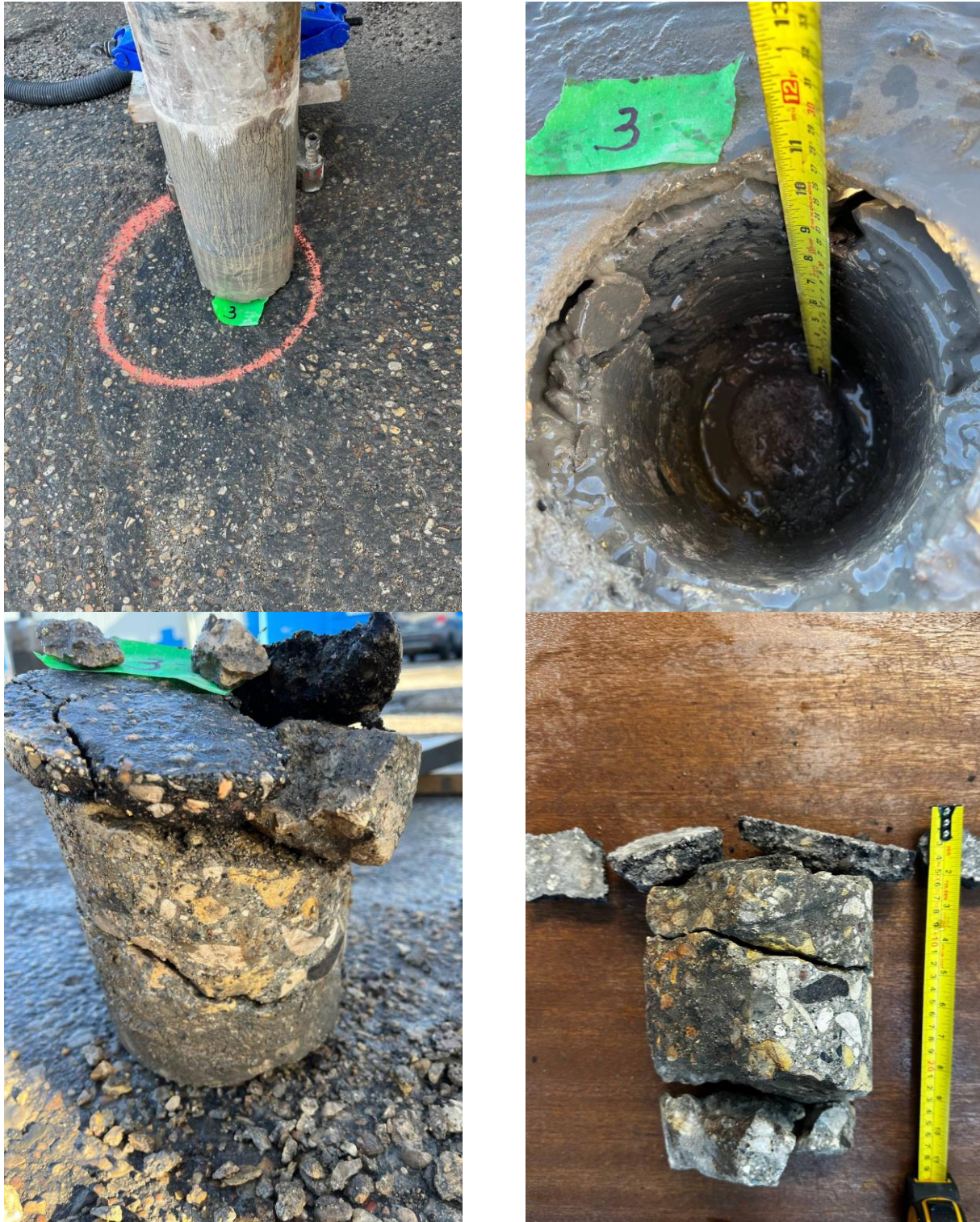
Figure 3. Photos showing Core 3 pavement showing shear stress deterioration of concrete and void between pavement and base surface
