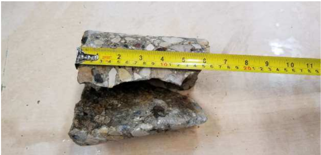
South bound transverse joint, Sta. 1+200
