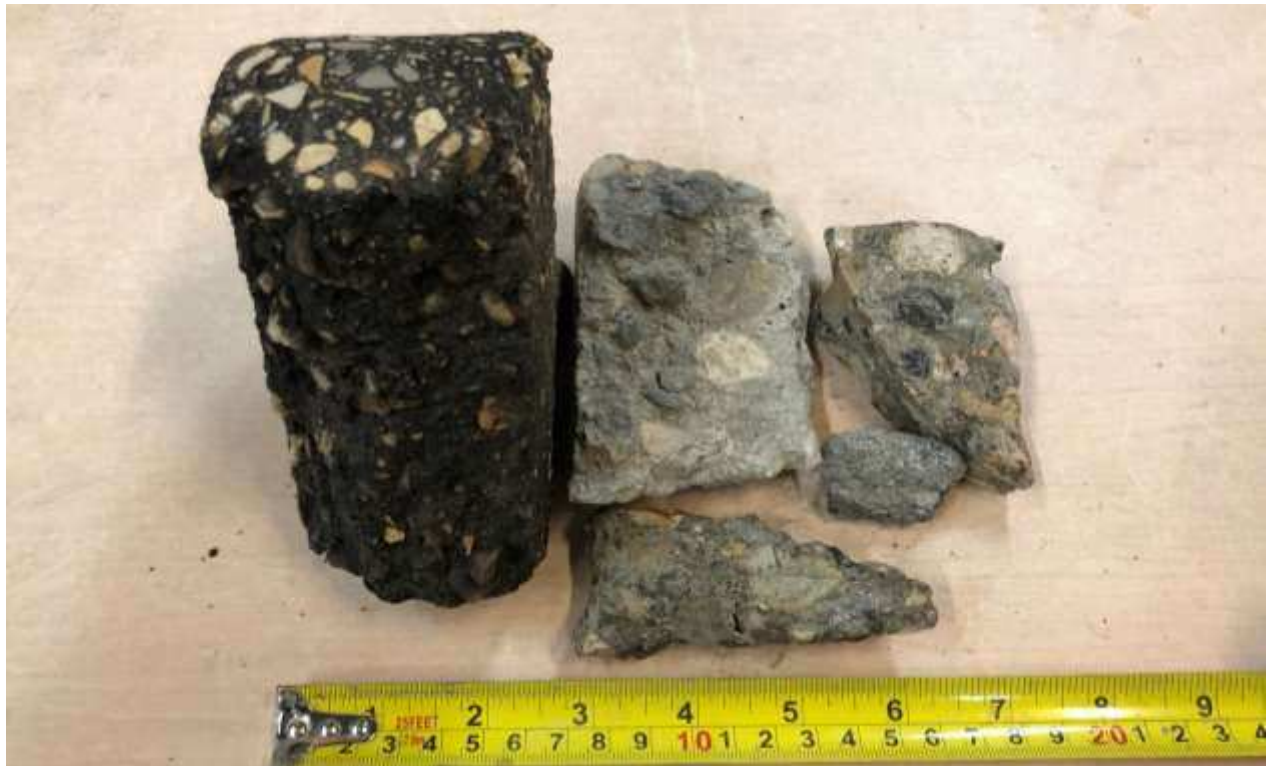
South bound transverse joint, Sta. 1+560
