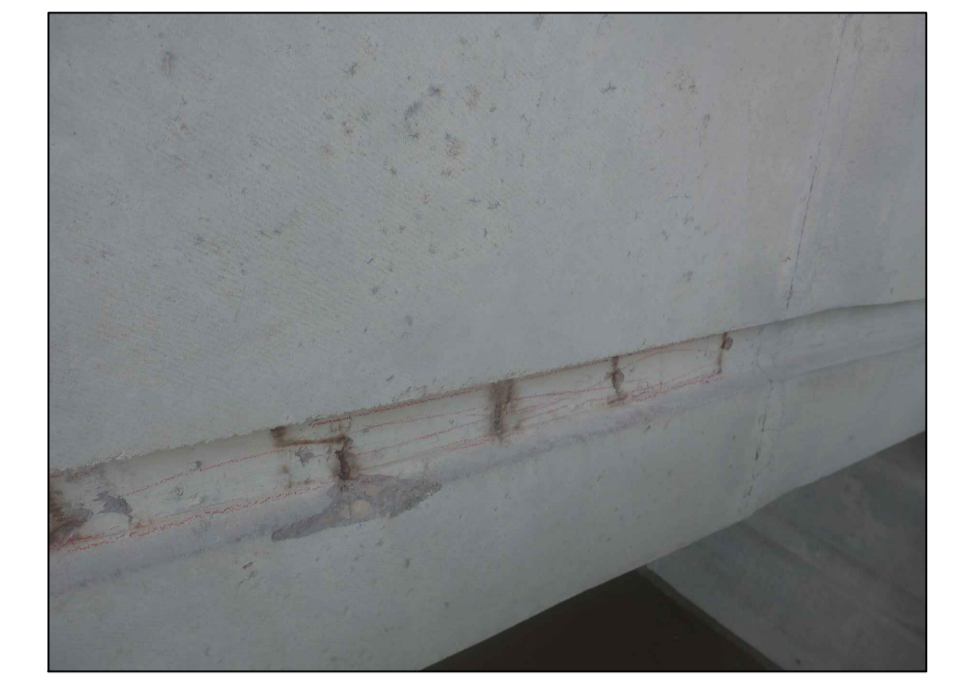
PHOTO 2 LOW COVER AND RUST STAINING
