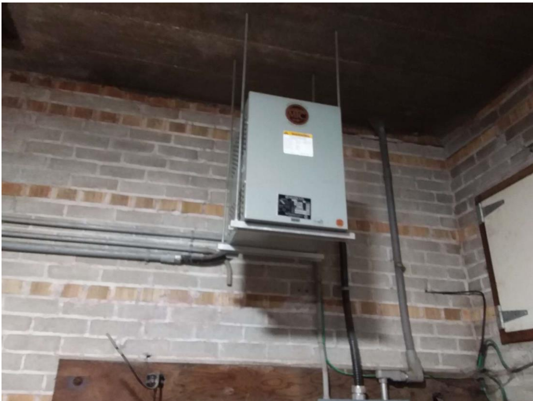
PCB, V0000(No), TRANSFORMER, Control/Motor Room (Location #: 1)
