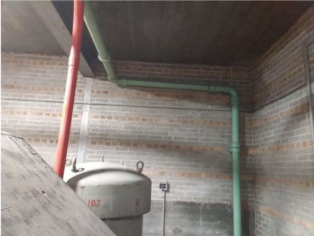
Pb Products, V9000(Yes), BELL AND SPIGOT FITTINGS, Rainwater leader, Control/Motor Room (Location #: 1)
