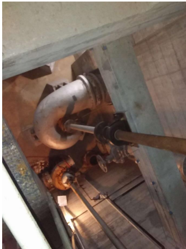
Pump Room (Location #: 2)
