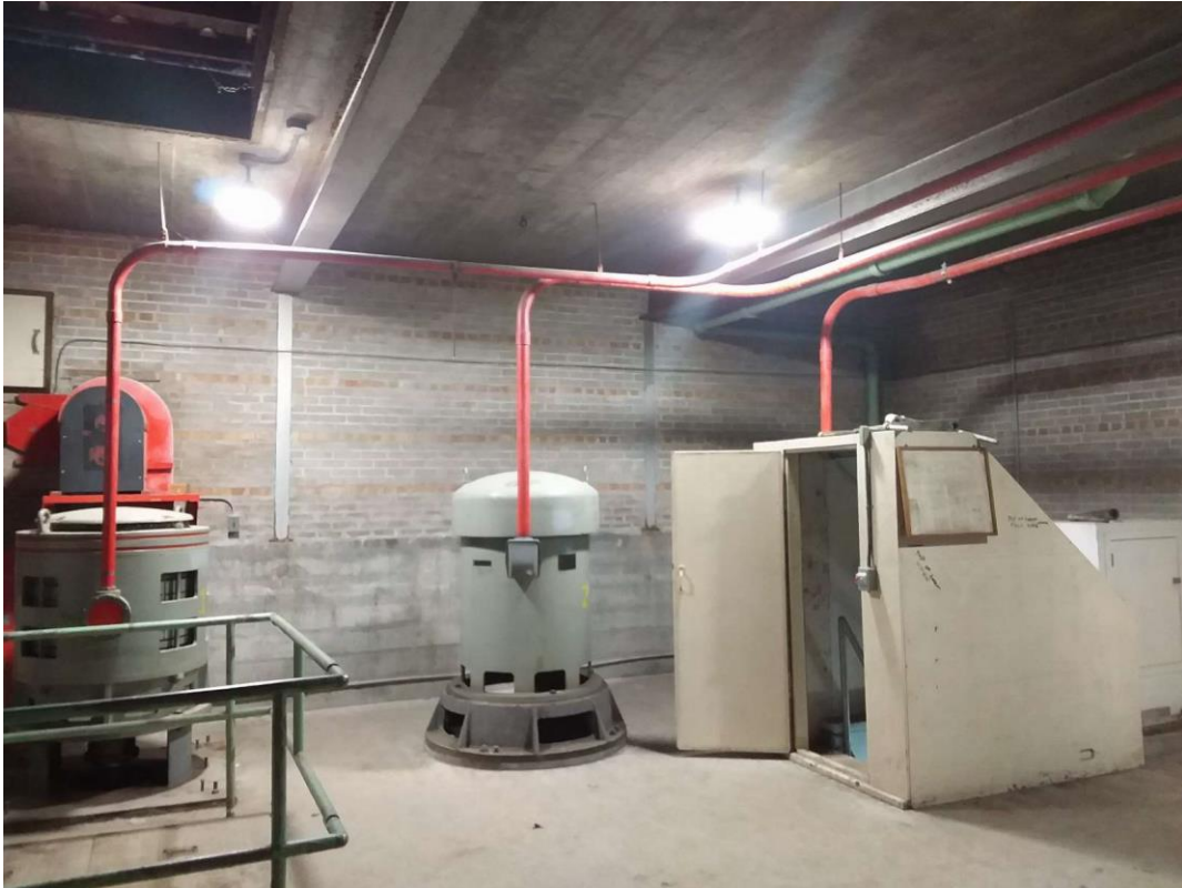
Control/Motor Room (Location #: 1)
