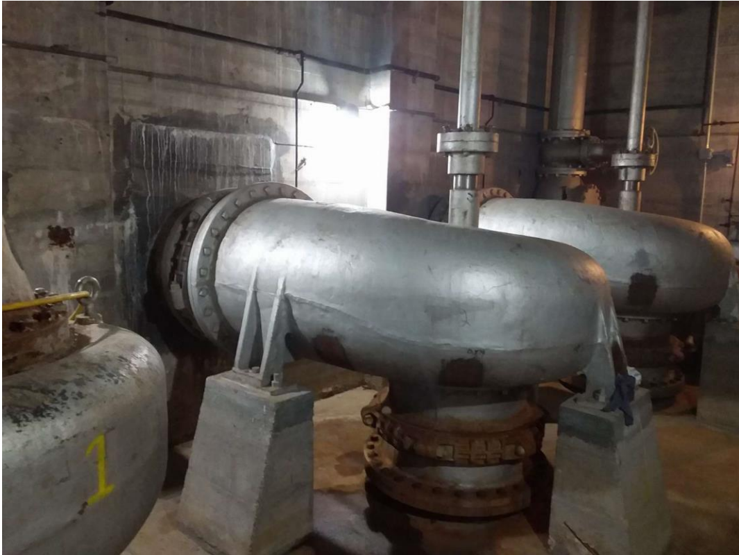
Mechanical Equipment, All, Not Insulated, Pump Room (Location #: 2)
