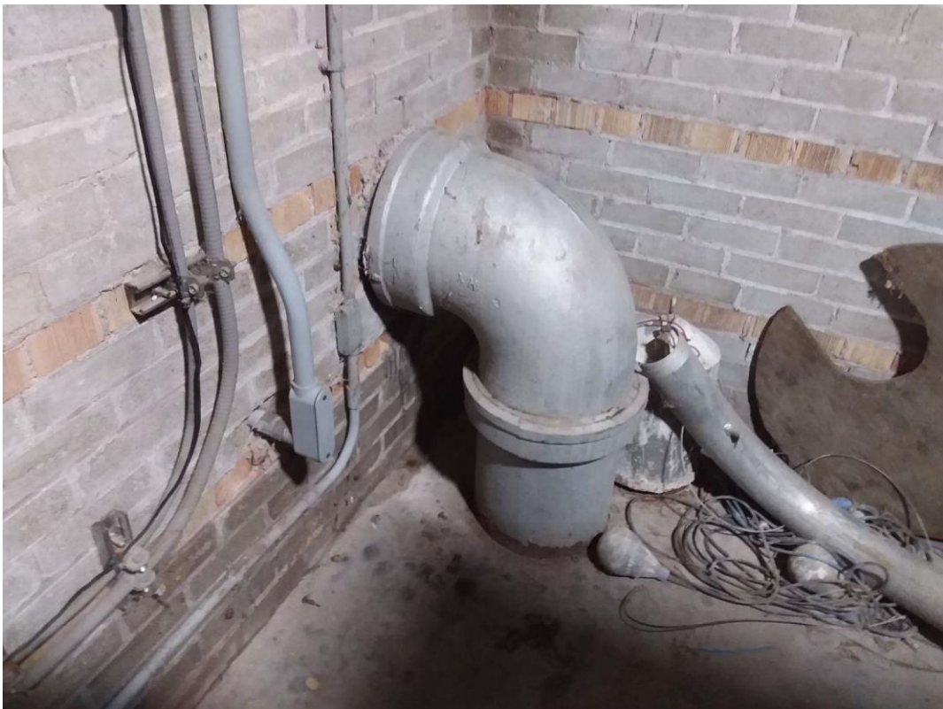
Pb Products, V9000(Yes), BELL AND SPIGOT FITTINGS, Rainwater leader, Control/Motor Room (Location #: 1)
