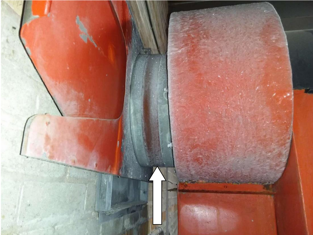
V9500 (Presumed Asbestos), Duct, Duct Connector, Textile, Control/Motor Room (Location #: 1) Red
