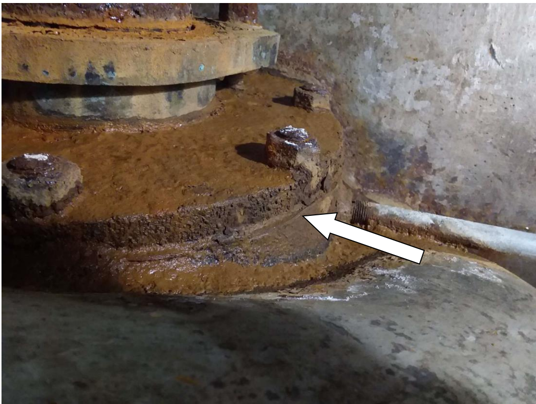
S0001A (None), Mechanical Equipment, Pump, Gasket, Pump Room (Location #: 2)
