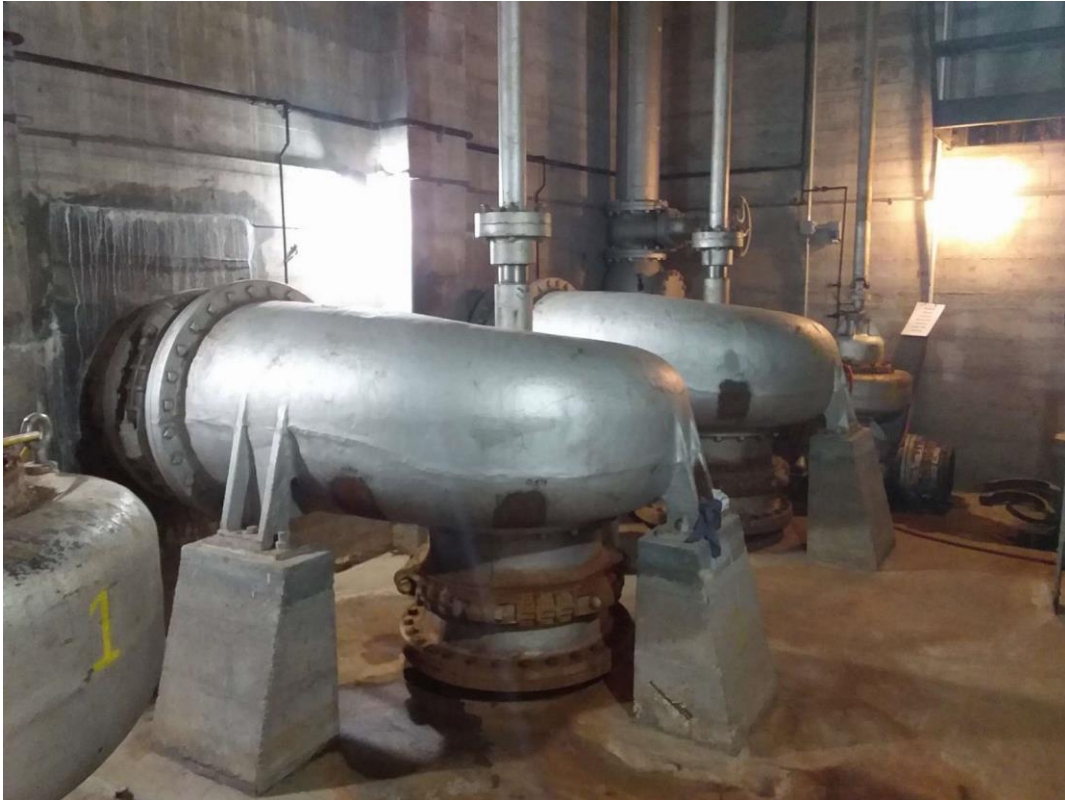
Pump Room (Location #: 2)
