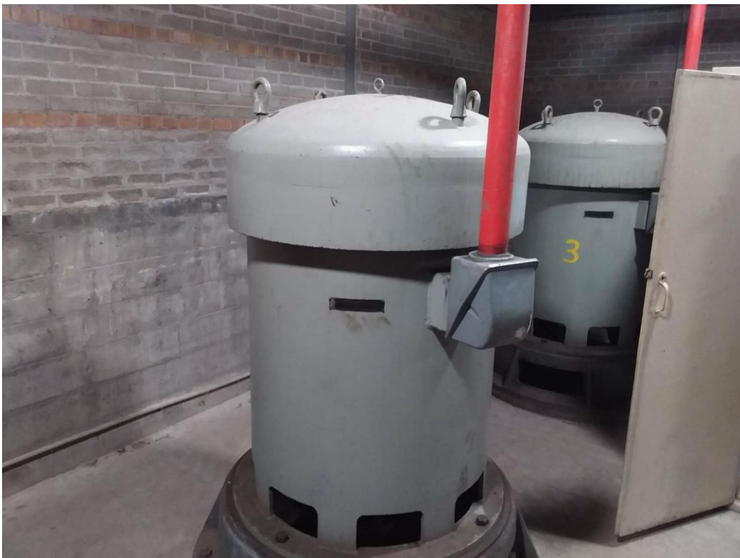
Mechanical Equipment, Not Insulated, Control/Motor Room (Location #: 1)
