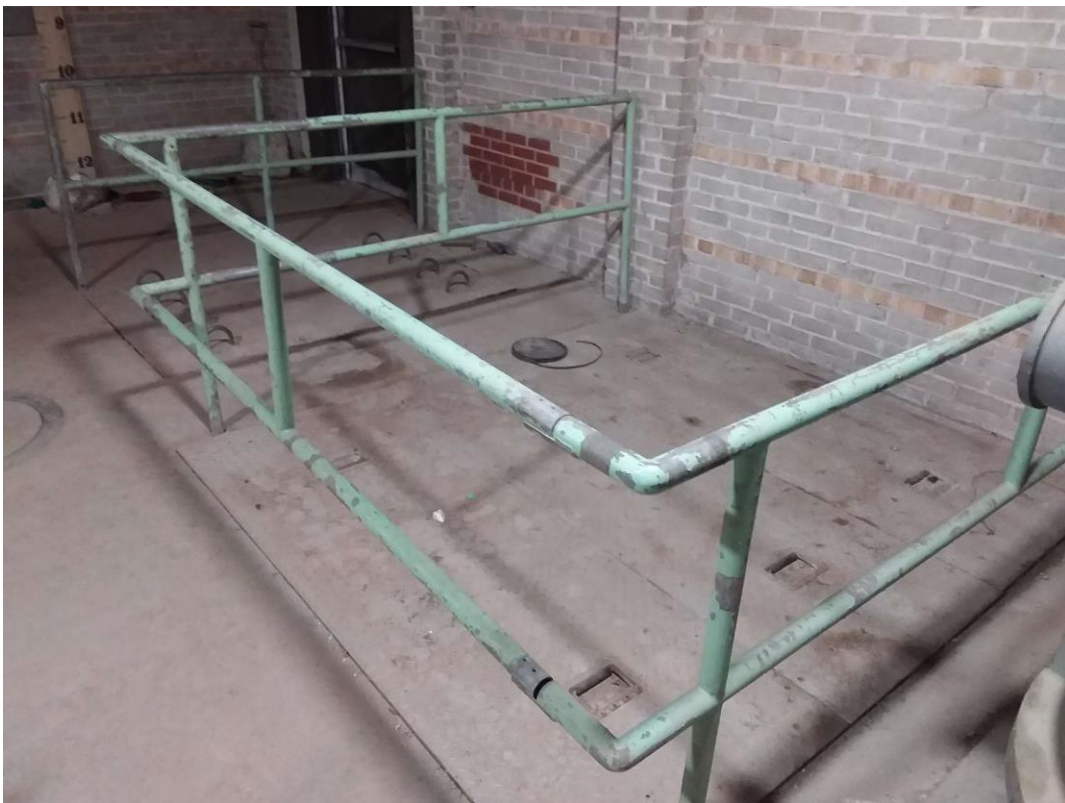
L0001(Lead, Yes), Green, Piping, Control/Motor Room (Location #: 1) Green - Handrail
