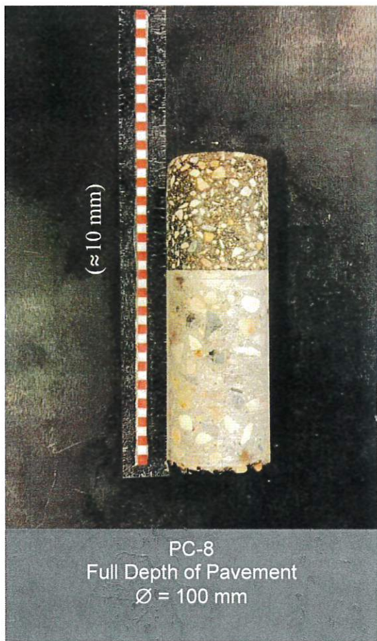
Photograph 8: Specimen from Ellie Avenue, Eastbound Curb Lane
