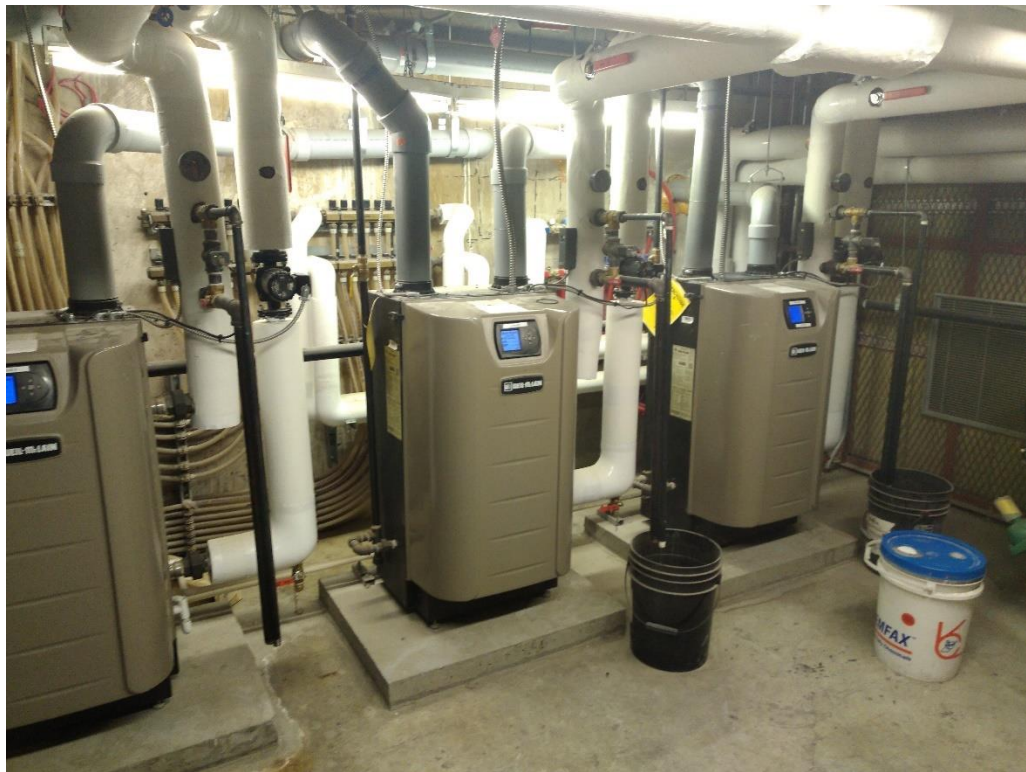
Figure 15: Boiler plant on Smith Street side of parkade.
