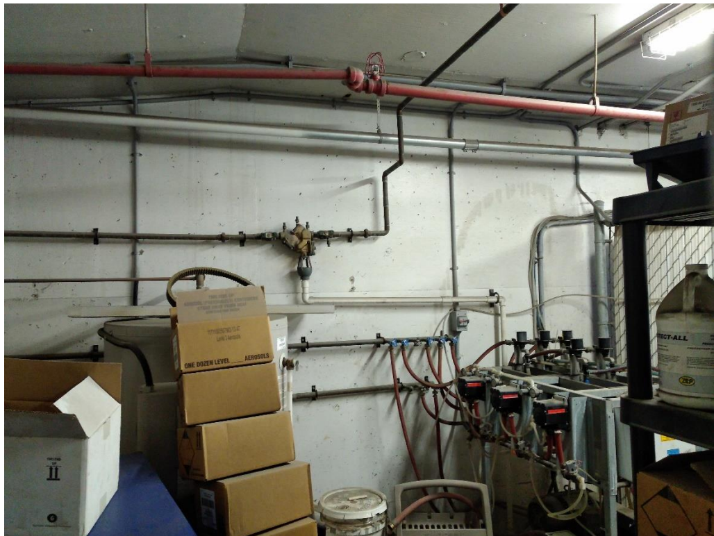
Figure 8: High pressure car wash pumps and dedicated hot water tank.
