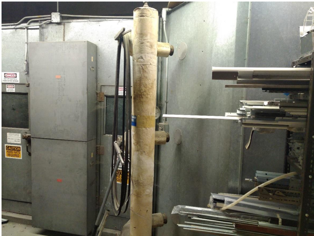
Figure 21: Capped glycol heat reclaim system.
