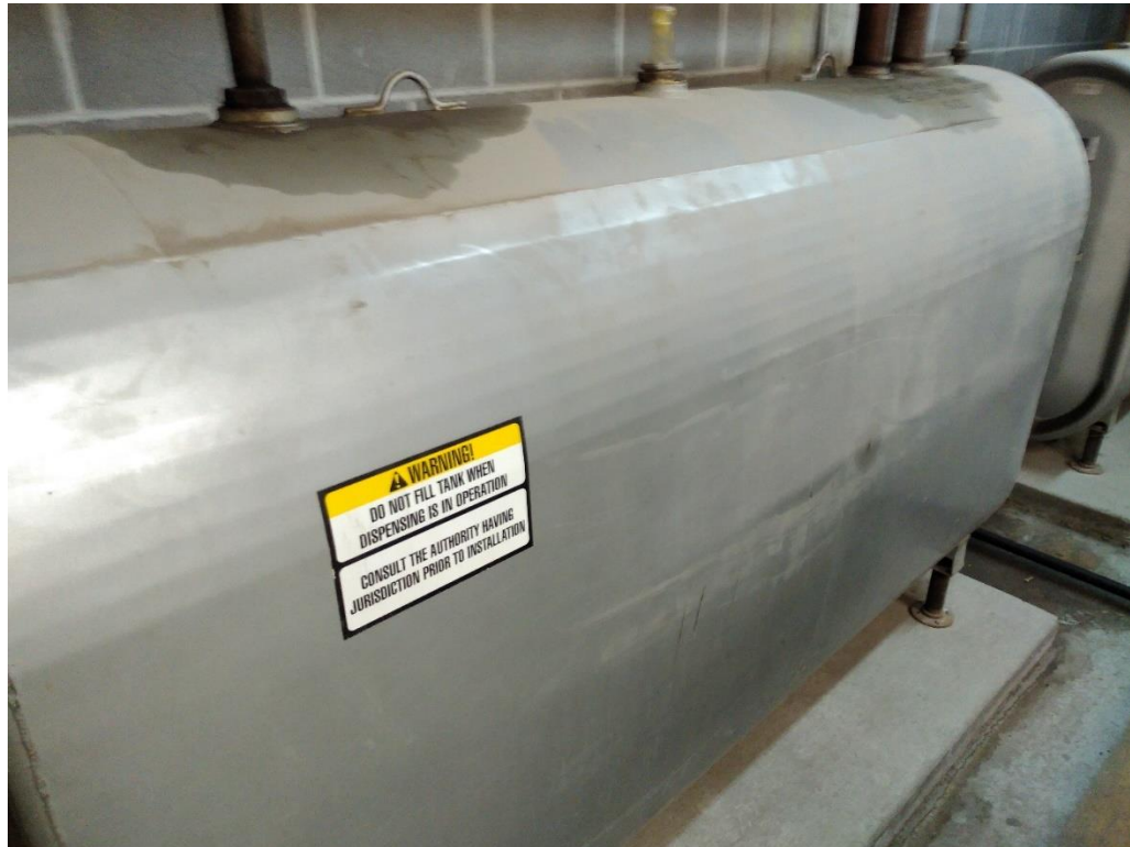
Figure 19: Double wall tank with signs of fuel oil leaking at tapings.
