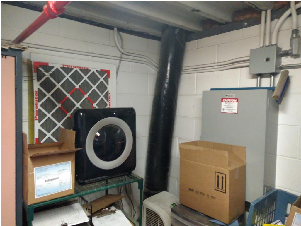
Figure 23: Intake and portable AC unit for Parking Authority office
