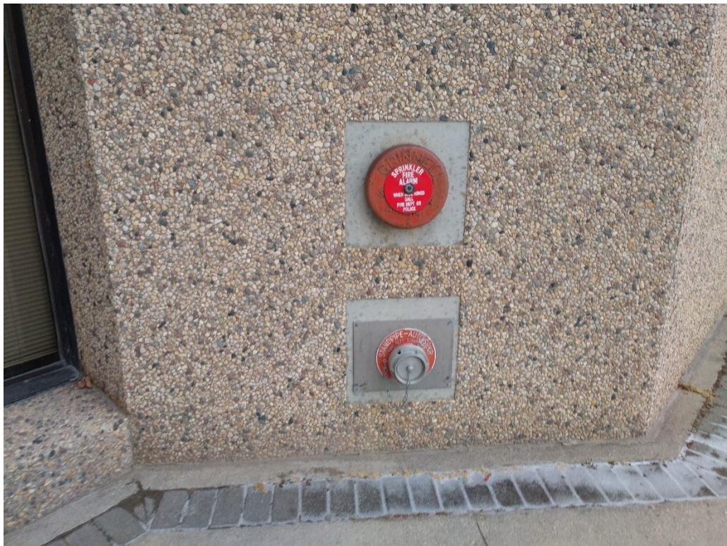
Figure 13: Fire department connection on building face.
