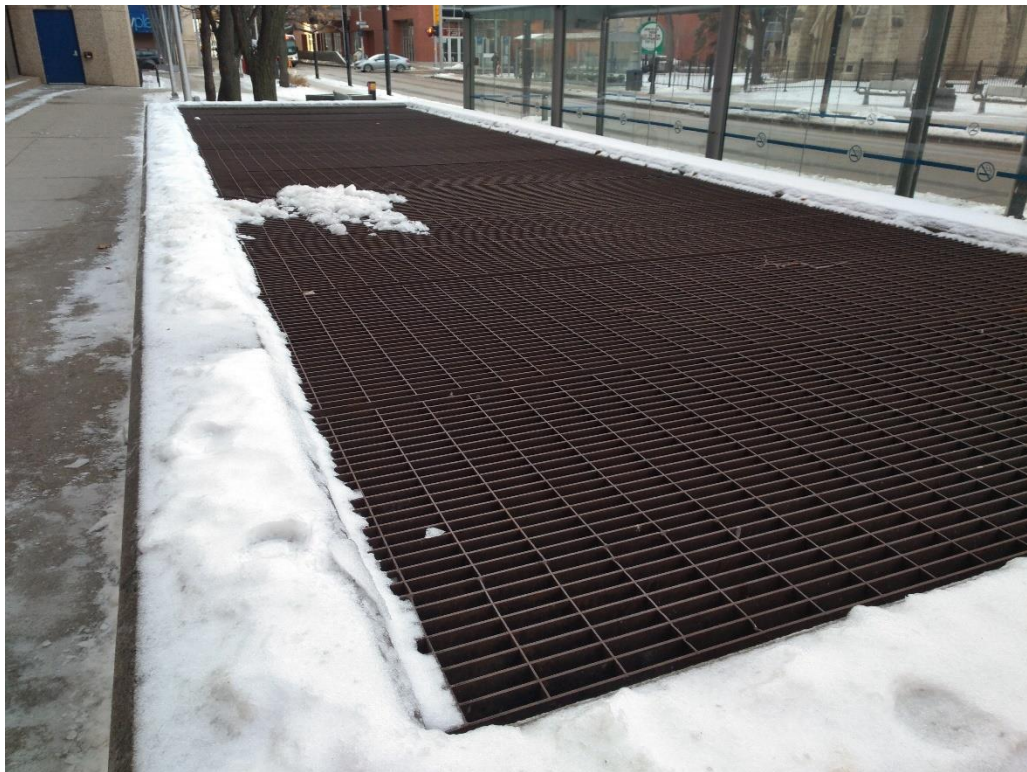
Figure 26: Intake louver for parkade make-up air unit.
