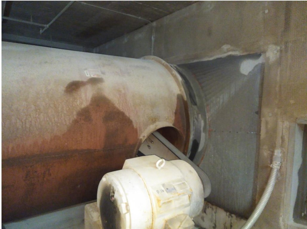
Figure 22: Exhaust fan serving parkade ventilation system.
