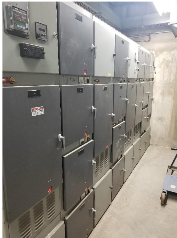
Figure 30: Part of the main distribution.
