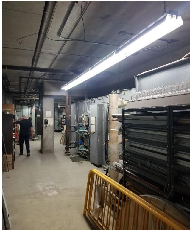
Figure 29: Back of house lighting
