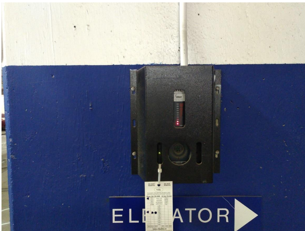
Figure 25: CO detector located on column in parkade.
