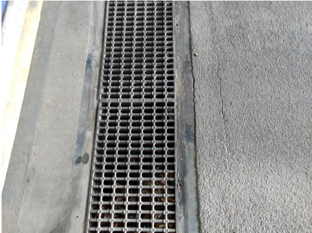
Figure 7: Trench drain on one of the four entrance ramps.
