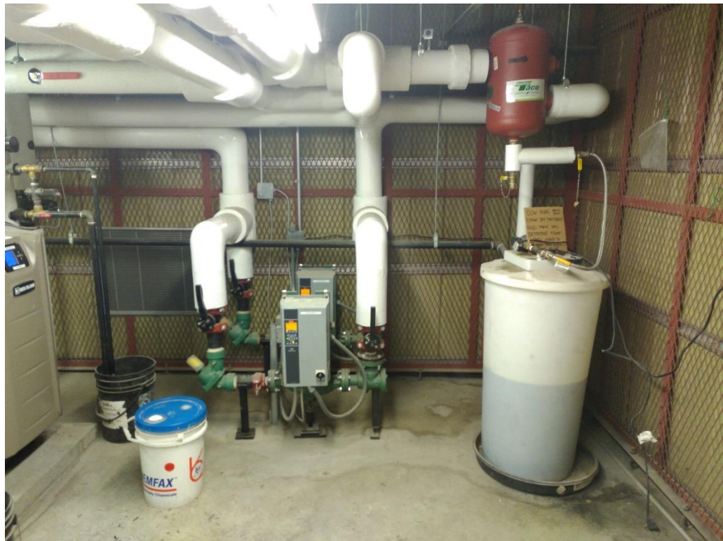
Figure 16: VFD driven pumps on hydronic system, in-line separator and glycol fill tank
