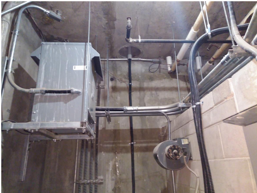
Figure 24 Exhaust fan not connected to anything in electrical room next to Parking Authority office.
