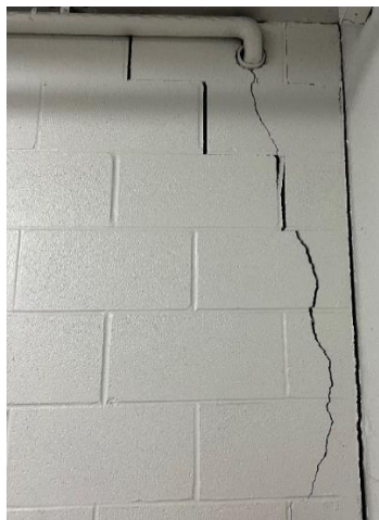
Figure 9: Vestibule Step Cracks
