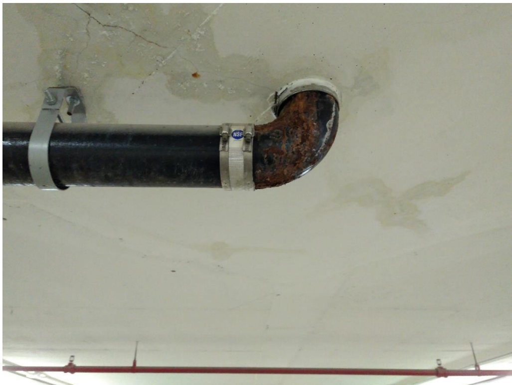
Figure 3: Localized corrosion on new cast iron pipe around drain.
