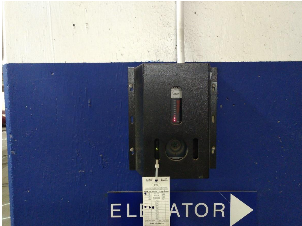
Figure 25: CO detector located on column in parkade.
