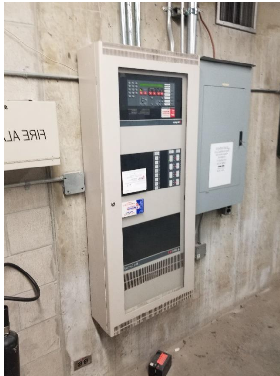
Figure 34: Main fire alarm panel
