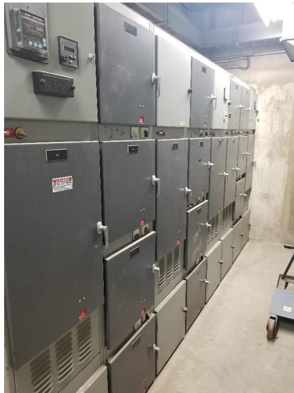
Figure 30: Part of the main distribution.
