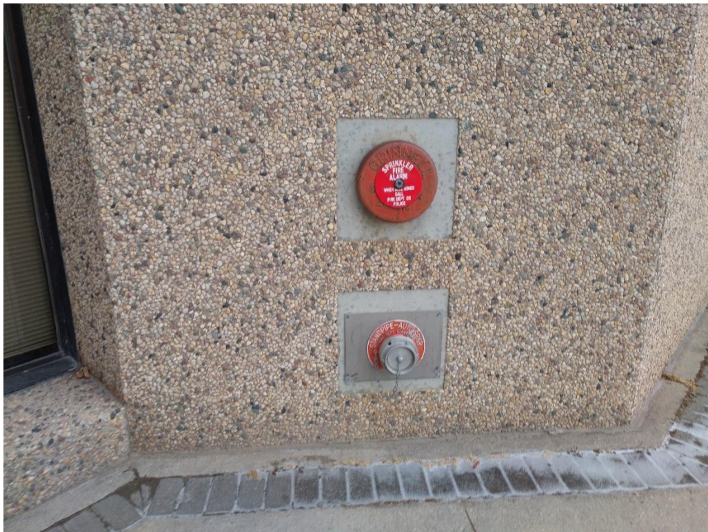
Figure 13: Fire department connection on building face.
