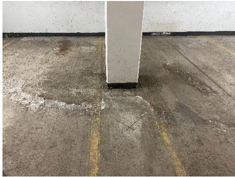
Figure 13: Staining around Column
