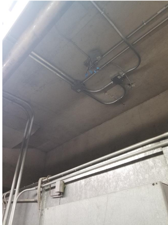
Figure 32: Junction box missing cover.
