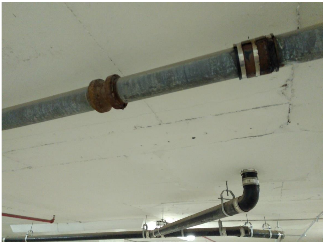
Figure 2: Galvanized discharge piping from lower level sump pits.
