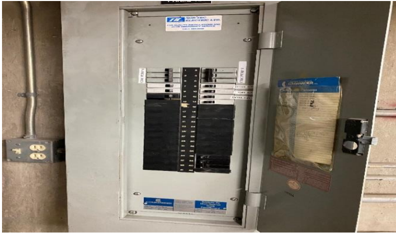
Figure 12: Indicate Essential Panelboard no longer used and obsolete Security Booth Panel
