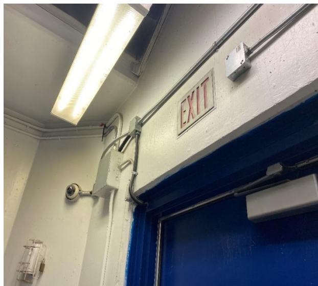
Figure 14: Exit Signs in Stairwells not functioning and improper style
