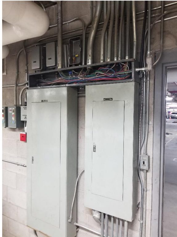
Figure 31: Wire-way missing cover
