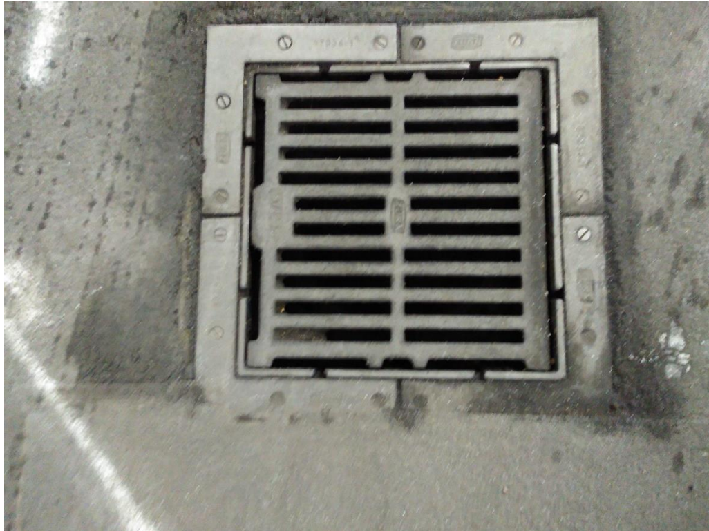
Figure 4: Galvanized drain on upper parkade level.
