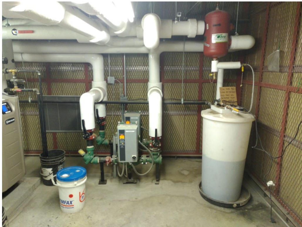
Figure 16: VFD driven pumps on hydronic system, in-line separator and glycol fill tank
