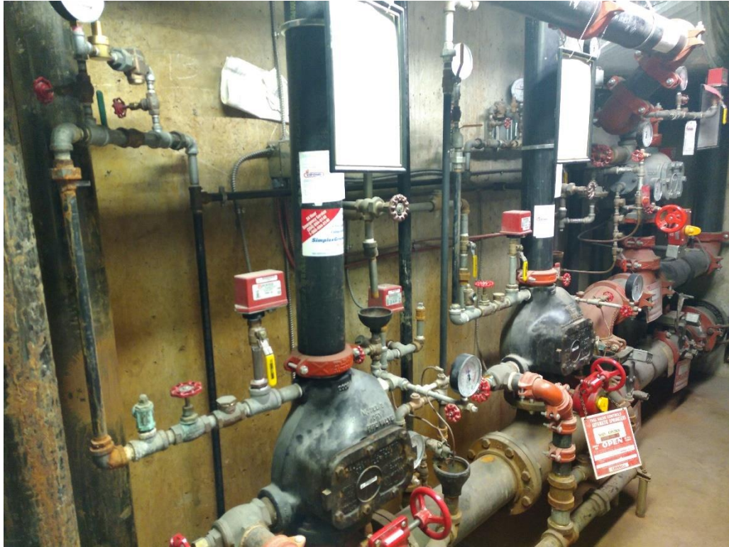
Figure 11: Sprinkler Header in Northeast service entrance room.
