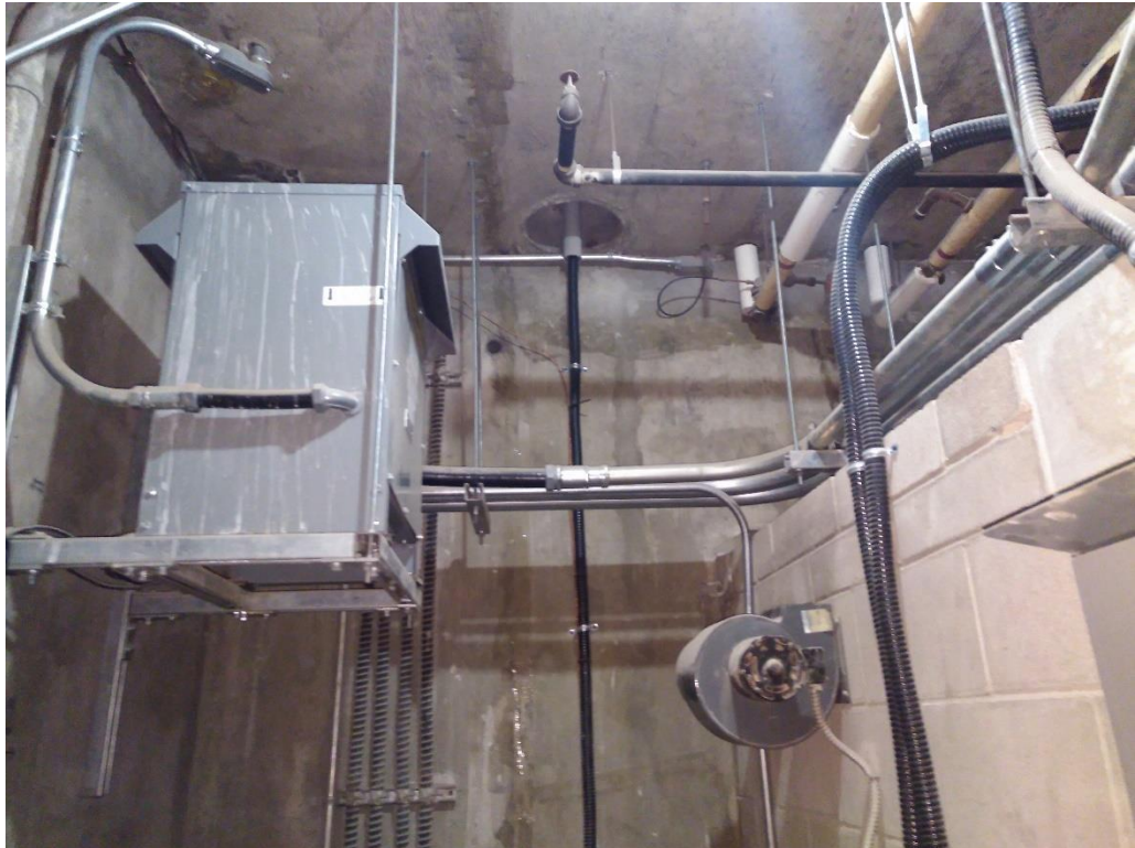
Figure 24 Exhaust fan not connected to anything in electrical room next to Parking Authority office.
