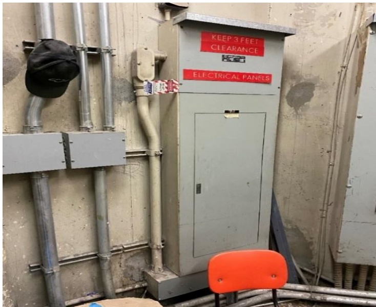
Figure 11: Indicate Essential Panelboard no longer used and obsolete Security Booth Panel
