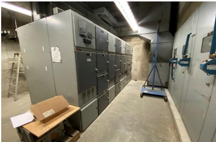
Figure 13: The Main 3000 Amp Westinghouse Shared Electrical Distribution
