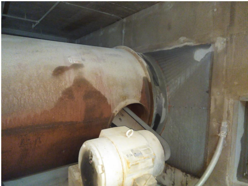
Figure 22: Exhaust fan serving parkade ventilation system.
