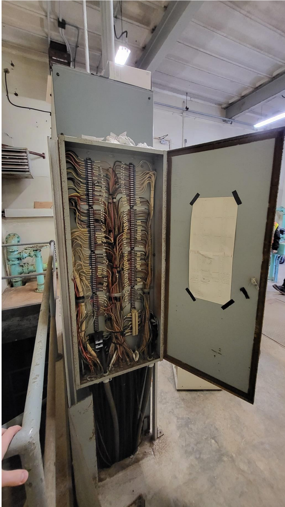
Photograph #5: Valve House Terminal Cabinet
