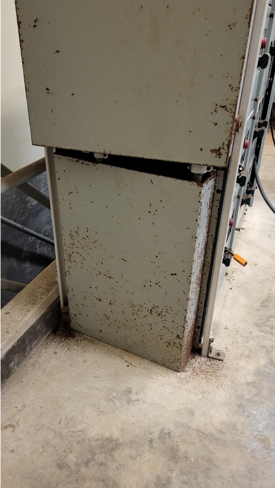
Photograph #2: Valve House Terminal Cabinet
