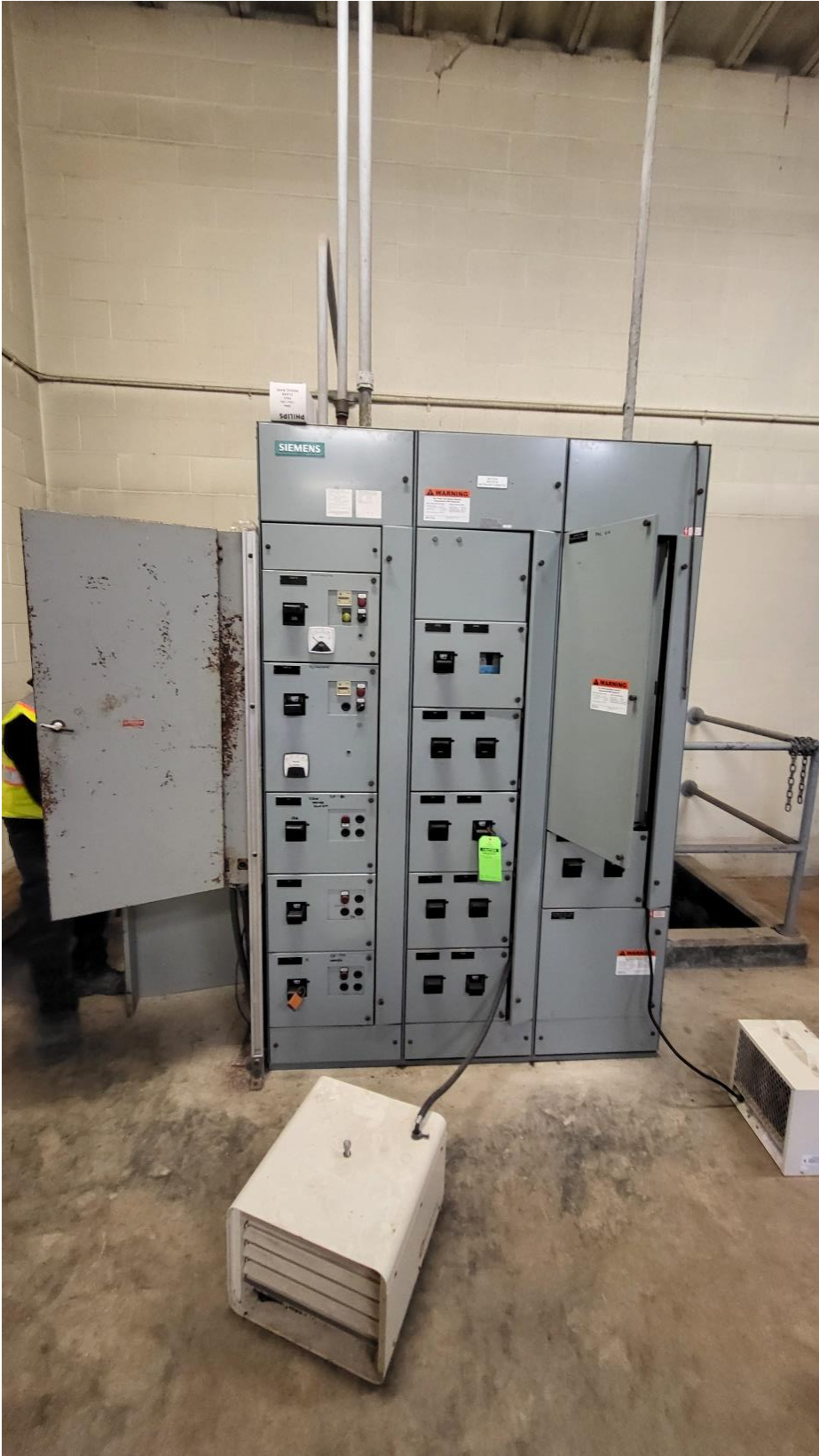
Photograph #4: Existing MCC in Maclean valve house, and temporary unit heater on the ground.
