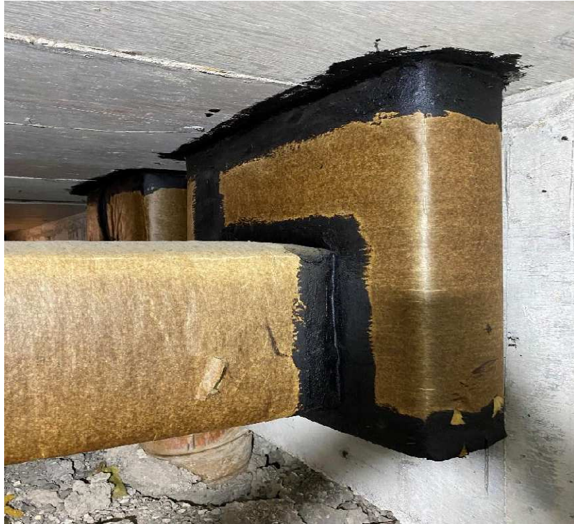
V9000, (Asbestos), Duct, black mastic, Crawlspace (Location # 22)
