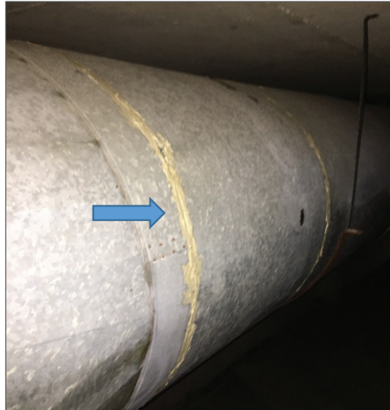
Photograph No. 26: Asbestos-containing beige mastic present on uninsulated ducting within the south crawlspace and basement board room (Samples 0008A-C).
