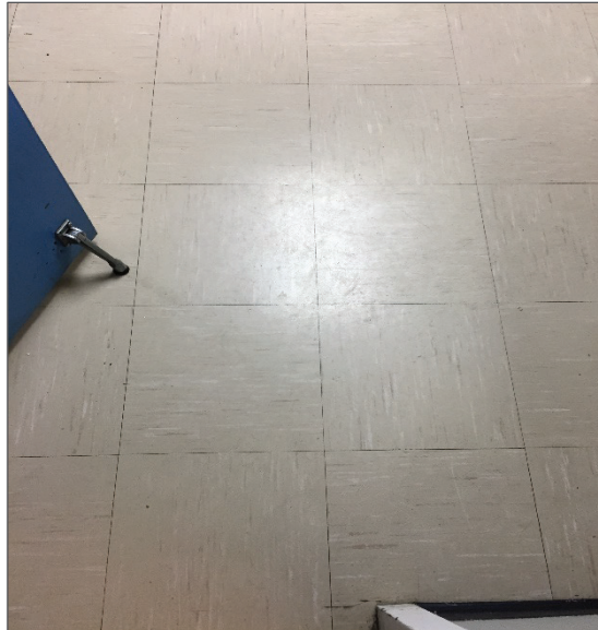
Photograph No. 18: Asbestos-containing vinyl floor tiles within the staff room Loc.59 (Samples 0046A-C).
