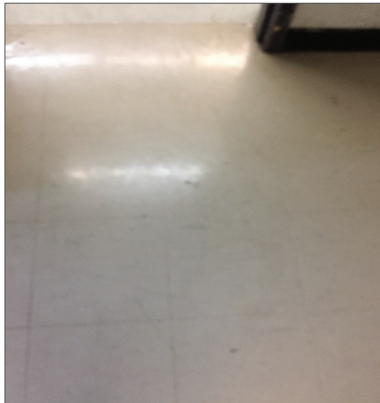
Photograph No. 17: Non-asbestos vinyl floor tiles within the corridors Loc.'s 52 and 58 (Samples 0038A-C).
