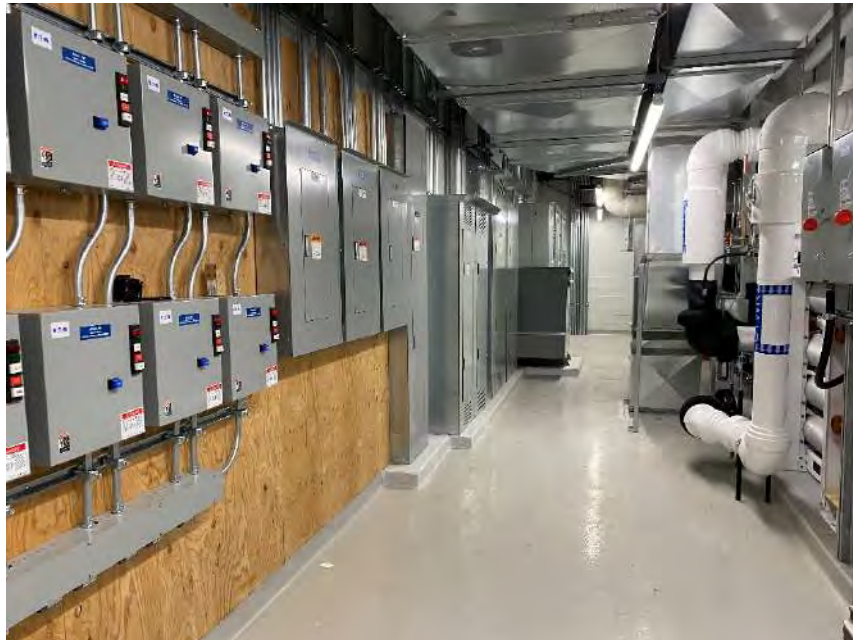
Photograph 28 – Interior, mechanical and electrical room Looking inward at the back area of the newly renovated mechanical and electrical room.
