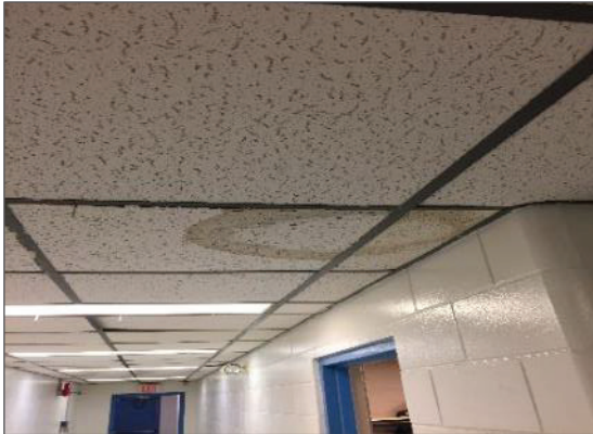
Photograph No. 28: Mouldy/water stained ceiling tiles in various locations.
