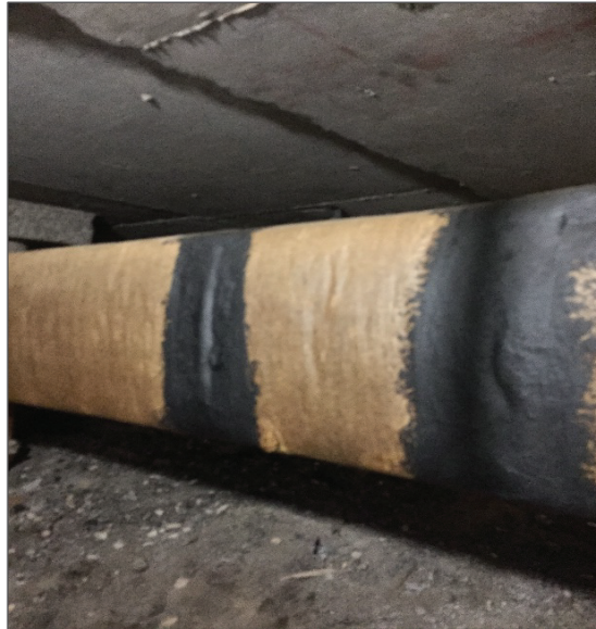
Photograph No. 24: Asbestos-containing black tar mastic on ducting within the south crawlspace (Samples 0007A-C).
