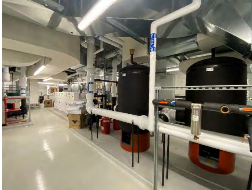
Photograph 27 – Interior, mechanical and electrical room Looking inward at the newly renovated mechanical and electrical room.
