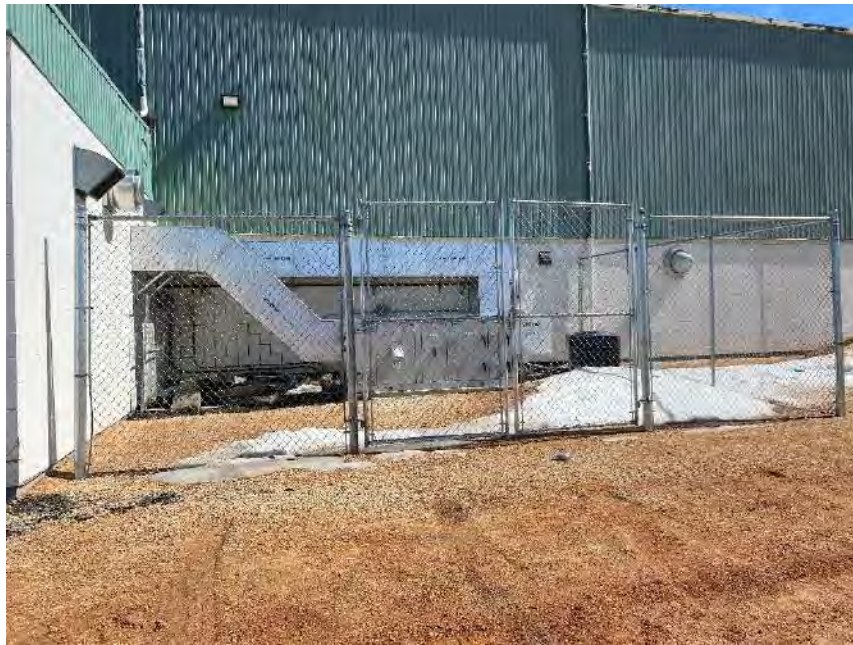
Photograph 40 – Exterior, air handling unit
