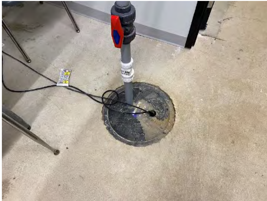
Photograph 42 – Interior, drain Looking at a drain located in the basement storage room.
