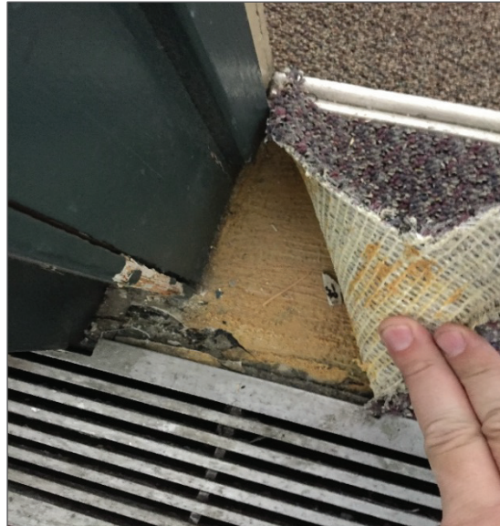
Photograph No. 20: Asbestos-containing vinyl floor tiles within the mezzanine board room and storage room under carpeting Loc.'s 66 and 67 (Samples 0053A-C).
