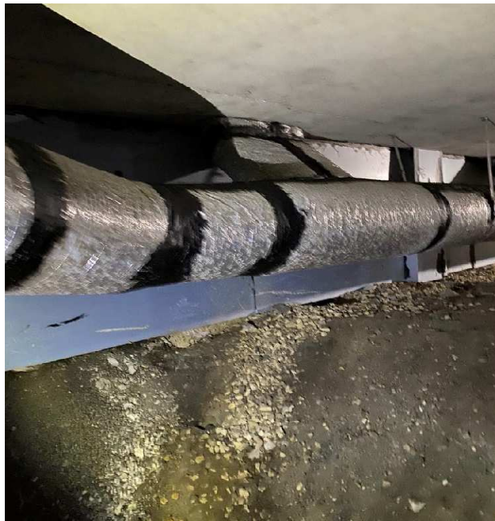
V9000, (Asbestos), Duct, black mastic, Crawlspace (Location # 22)
