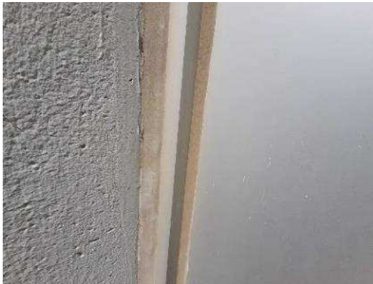
S0012A (None), Wall, Caulking, Exterior Of Building (Location #: 19)
