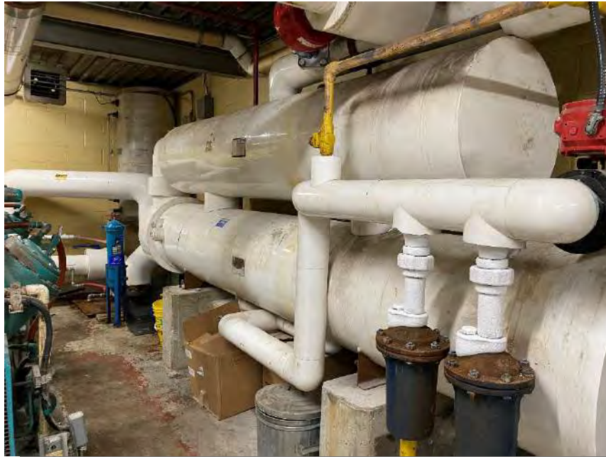
Photograph 37 – Interior, ammonia tanks Looking at ammonia tanks stored to the north of the Arena.
