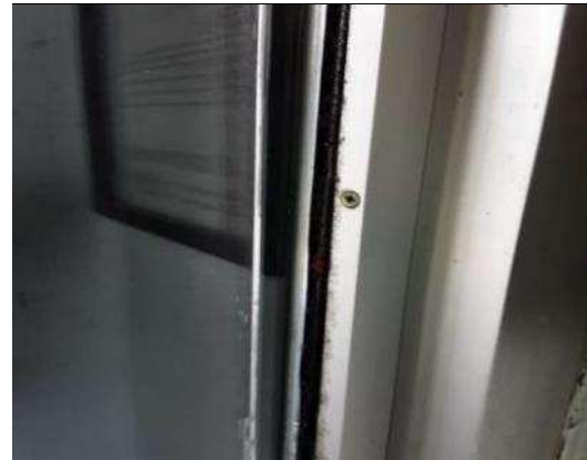
P0002 (None), Caulking, Foyer (Location #: 15)
