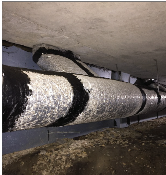
Photograph No. 25: Asbestos-containing black tar mastic on ducting within the south crawlspace (Samples 0009A-C).
