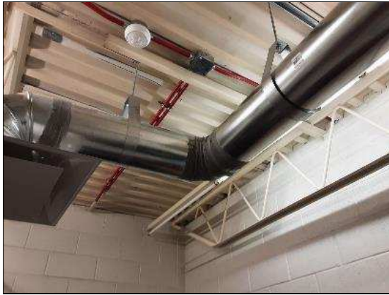
V0000 (None), Duct, Mastic, Grey, Storage Room (Location #: 3)
