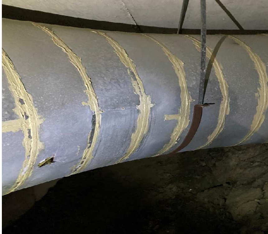
V9000, (Asbestos), Duct, beige mastic, Crawlspace (Location # 22)
