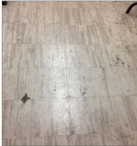
Photograph No. 12: Asbestos-containing vinyl floor tiles within the rink sound room Loc.15 (Samples 0023A-C).
