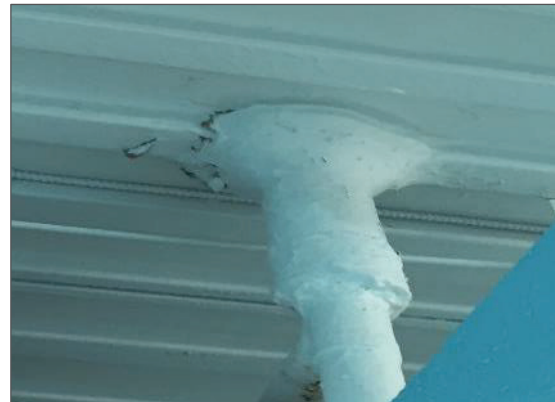
Photograph No. 2: Asbestos-containing parging cement on rain water leader fittings.
