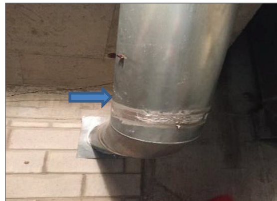
Photograph No. 22: Non-asbestos grey mastic on uninsulated ducting throughout the building.
