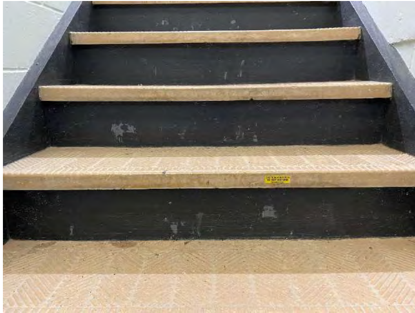
Photograph 43 – Interior, stairs leading to the second floor Looking at potentially asbestos containing materials on the stairs leading to the second floor.
