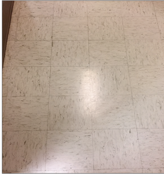
Photograph No. 16: Asbestos-containing vinyl floor tiles within the auditorium and adjacent rooms Loc.48 (Samples 0039A-C).
