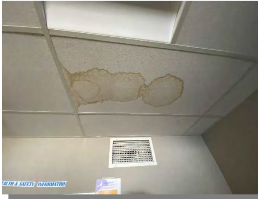
Photograph 41 – Interior, ceiling stain Looking at water damage stains on the ceiling of the staff kitchen that is to be removed.
