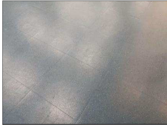
V0000 (None), Floor, Matt Flooring, Foyer (Location #: 15)
