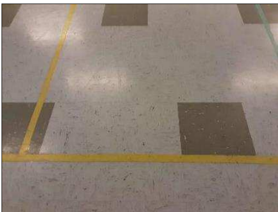
V9000 (Confirmed Asbestos), Floor, Vinyl Floor Tile and Mastic, Auditorium (Location #: 1)
