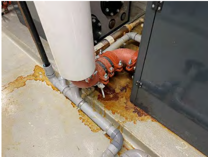
Photograph 44 – Interior, boiler room Looking at unknown stains located in the boiler room floor.
