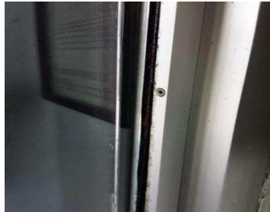
S0009C (None), Other, Caulking, Foyer (Location #: 15)
