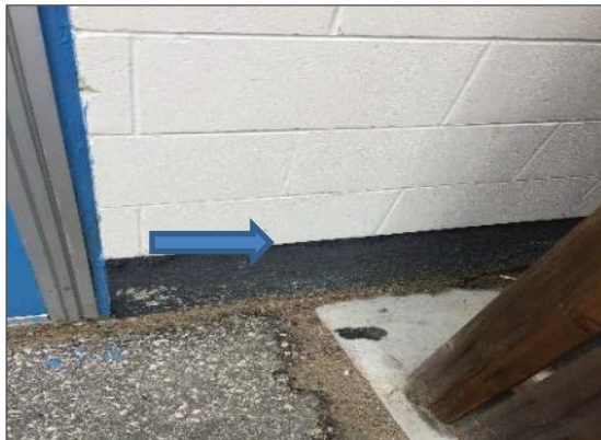
Photograph No. 27: Asbestos-containing stucco on lower exterior walls (Samples 0055A-C).
