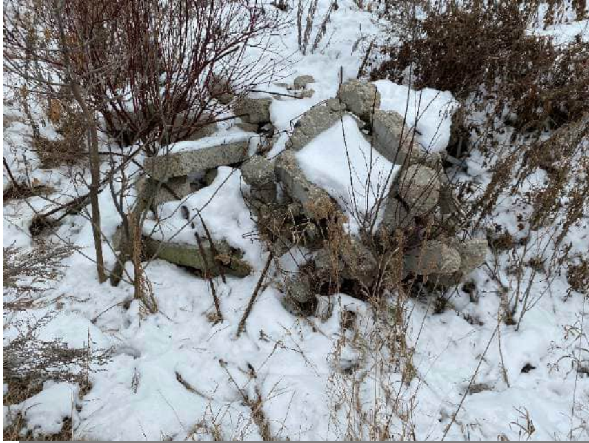
Photograph 29 – Concrete with Rebar
