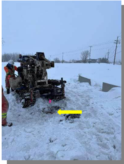
Photograph 1 – Northeast portion of the Site Looking west at the location of monitoring well MW01 (yellow arrow).
