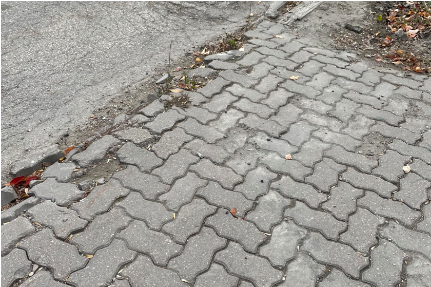
Figure 15. Pavers in poor condition.
