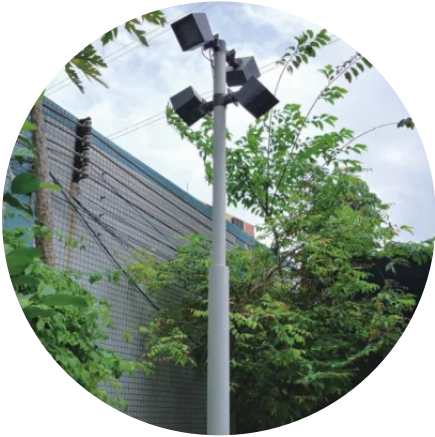
Figure 36. Modified street light with adjustable fixtures on existing base
