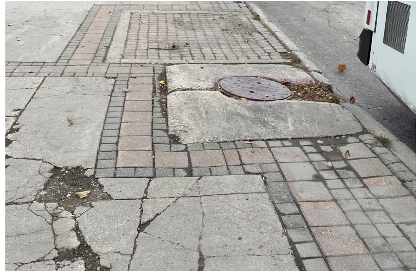
Figure 20. Poor sidewalk condition.
