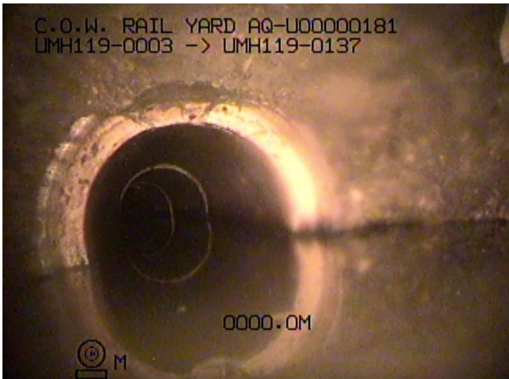
Figure 14 – AQ-U00000181 (GWWD Railyard) void around missing underdrain
