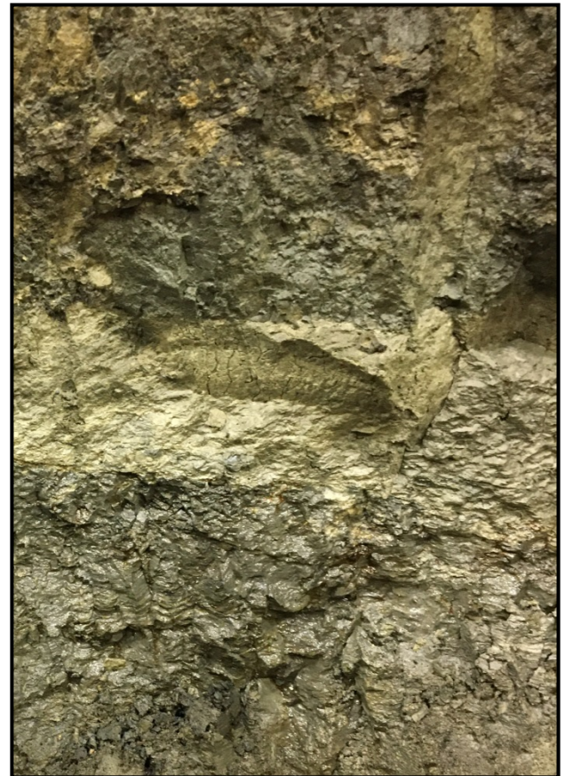
PHOTOGRAPH #2: Oily surface on the soil at S27 at approximately 2.0 metres below grade.
