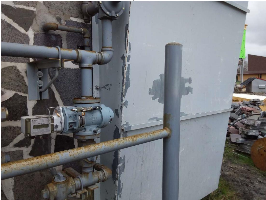
L0006(Lead, None), Grey, Duct, Generator Building (Location #: 3) Grey
