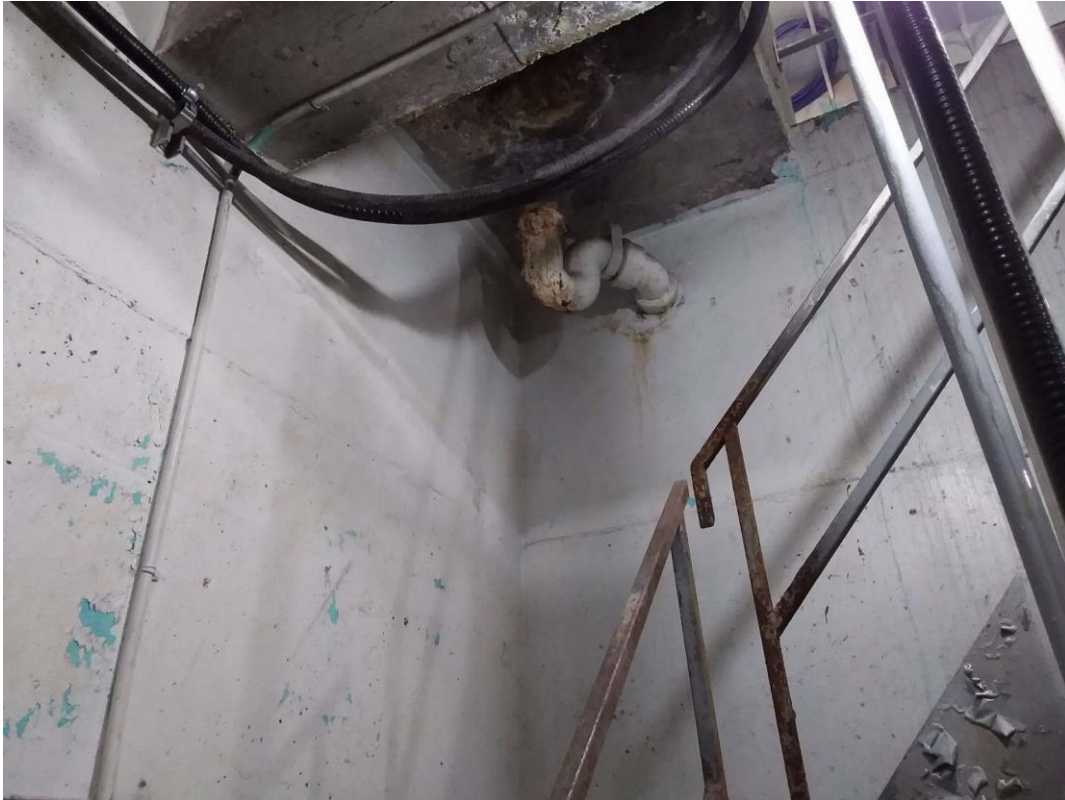
Pb Products, V9000(Yes), BELL AND SPIGOT FITTINGS, Motor Room (Location #: 1)
