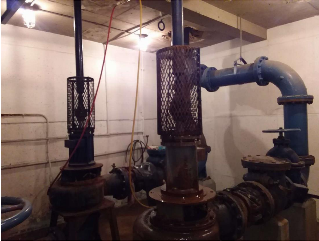
Pump Room (Location #: 4)
