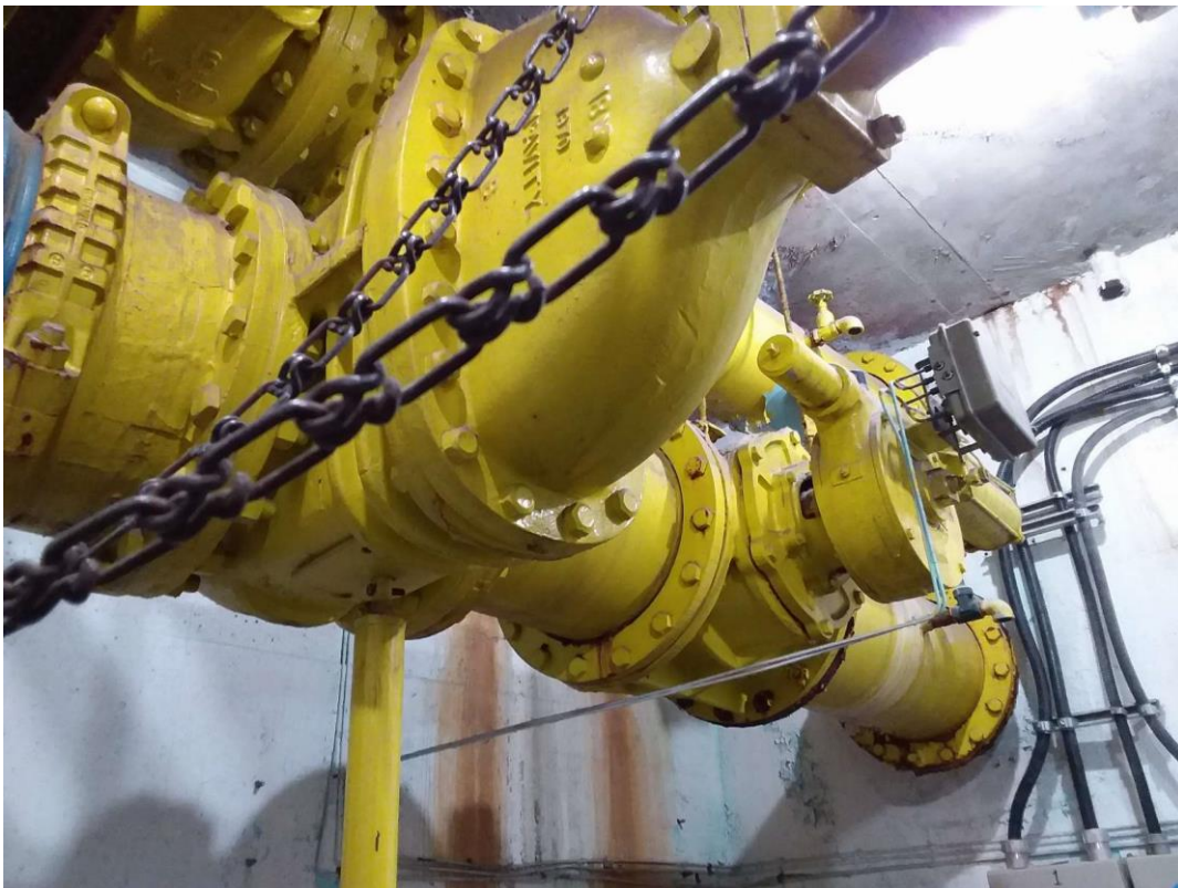
L0003(Lead, Yes), Yellow, Piping, Motor Room (Location #: 1) Yellow
