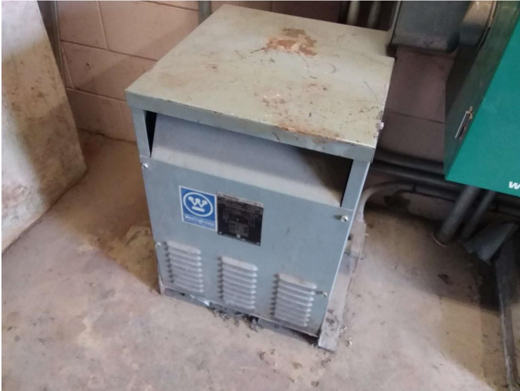
PCB, V0000(No), TRANSFORMER, Generator Building (Location #: 3)
