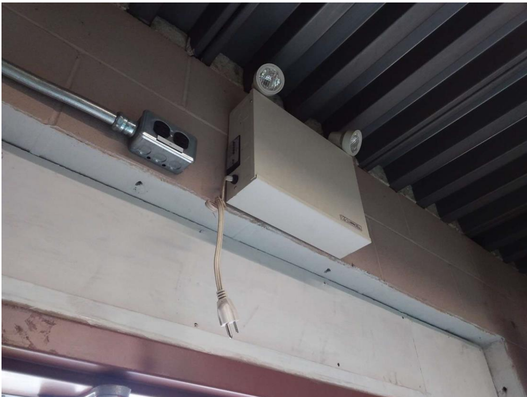
Pb Products, V9000(Yes), BATTERIES IN EMER. LIGHTS, Generator Building (Location #: 3)
