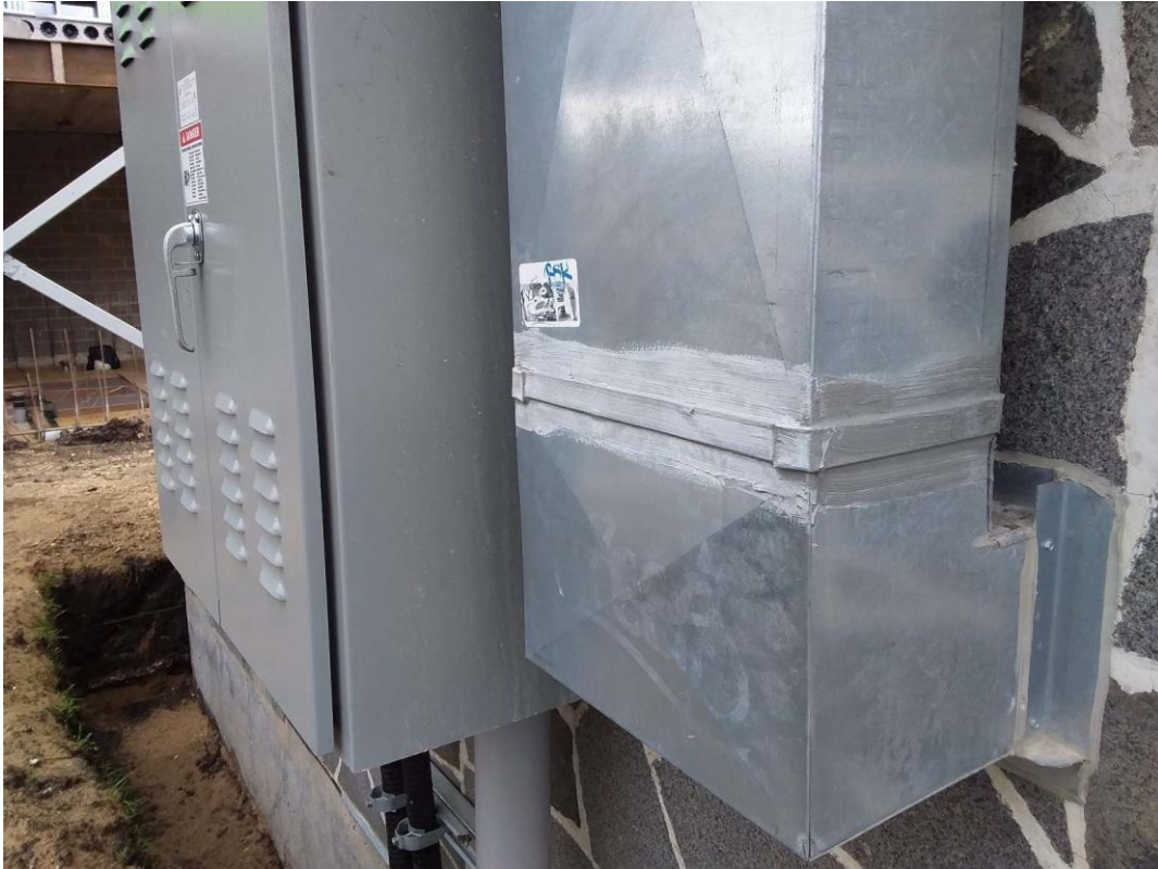
S0001 (None), Duct, Mastic, Grey, Generator Building (Location #: 3)
