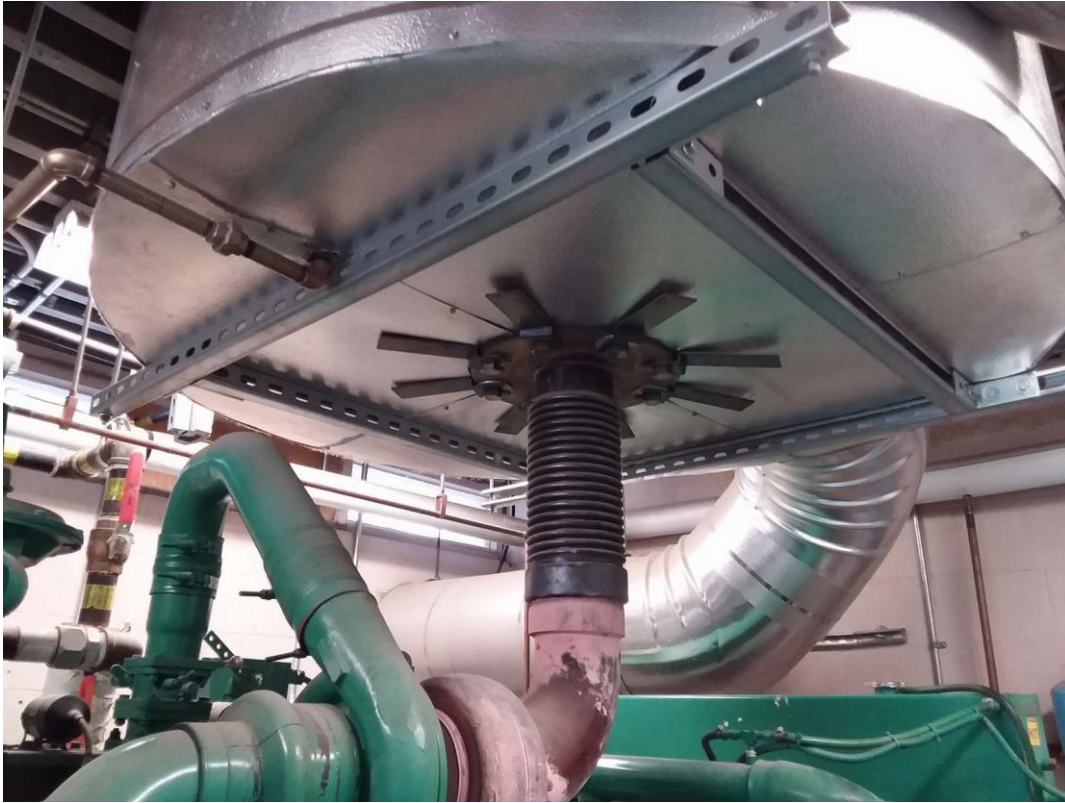
Duct, Exhaust, Not Insulated, Generator Building (Location #: 3)
