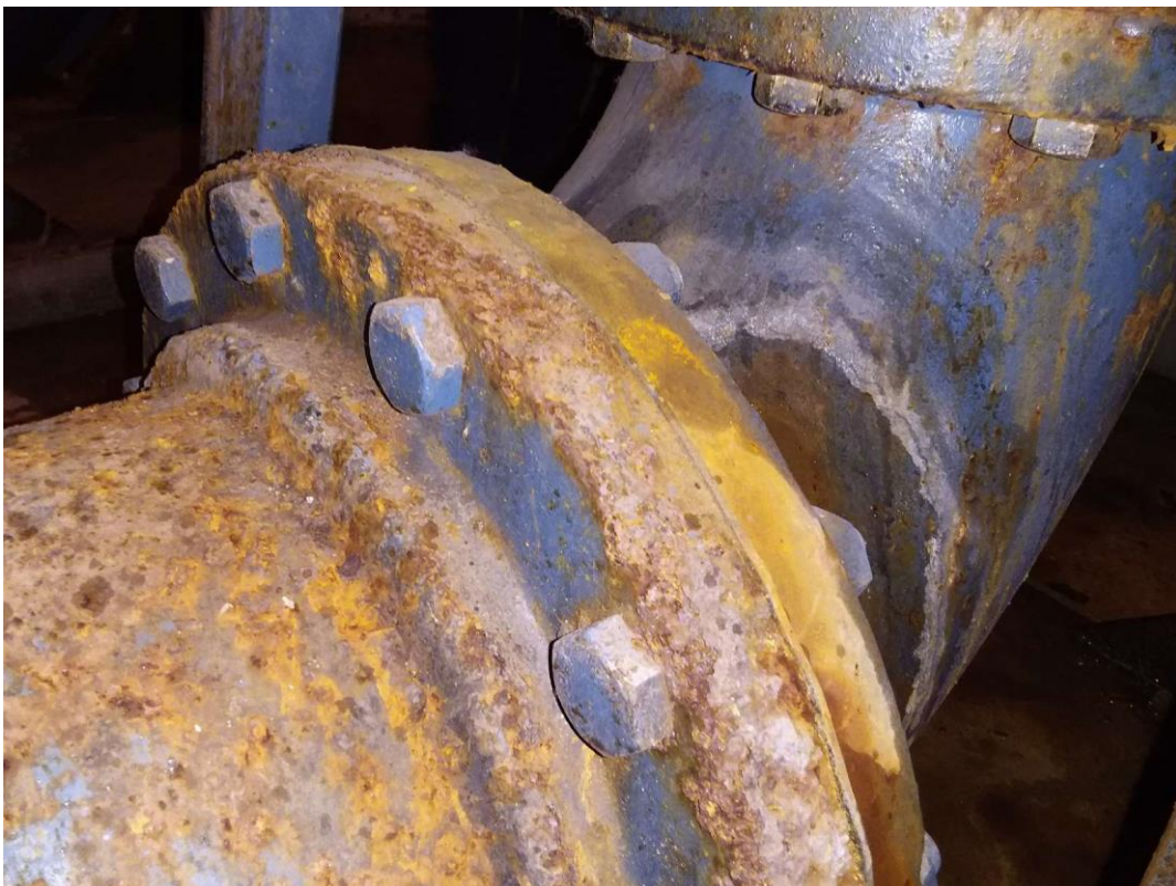
S0003A (None), Mechanical Equipment, Pump, Gasket, Pump Room (Location #: 4)
