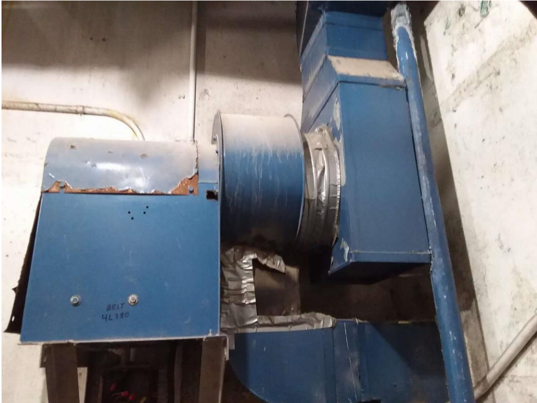
V9500 (Presumed Asbestos), Duct, Duct Connector, Textile, Motor Room (Location #: 1)
