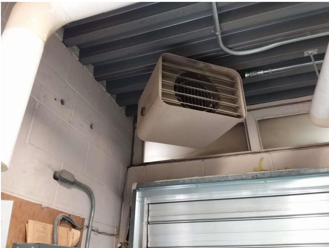
Mechanical Equipment, Unit Heater, Not Insulated, Generator Building (Location #: 3)
