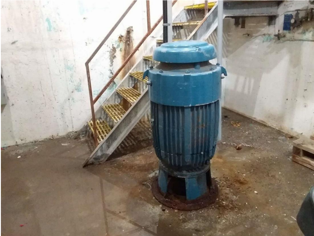
L0002(Lead, Yes), Blue, Mechanical Equipment, Motor Room (Location #: 1) Blue
