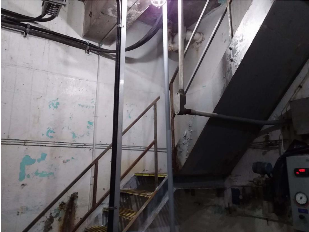
L0004(Lead, None), Silver, Floor, Motor Room (Location #: 1) Silver, stairs
