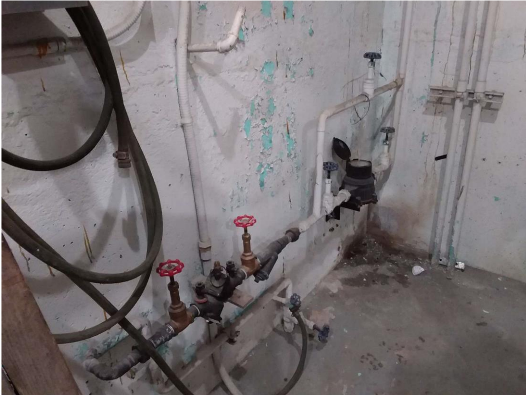
Piping, All, Not Insulated, Motor Room (Location #: 1)
