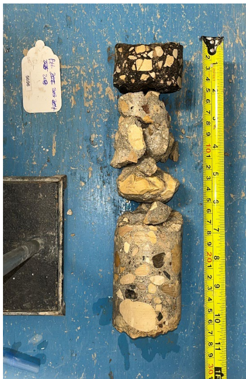
Figure 17 – Core Sample No. 208 – Mountain Ave
