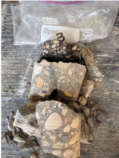
Core 3 - Joint (Deteriorated)
