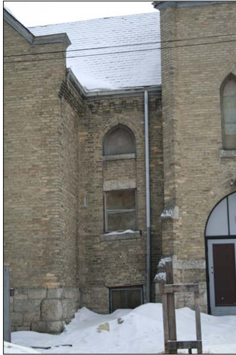
West façade detail showing settling and cracks, 2009
