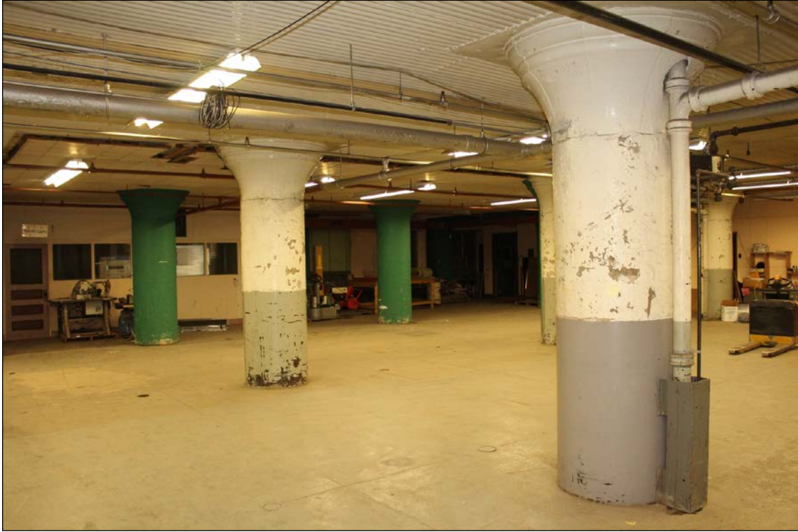
Plate 15 – J.R. Watkins Company Warehouse, 90 Annabella Street, ground floor columns and corrugated ceiling, 2016. ( M. Peterson, 2016. )
