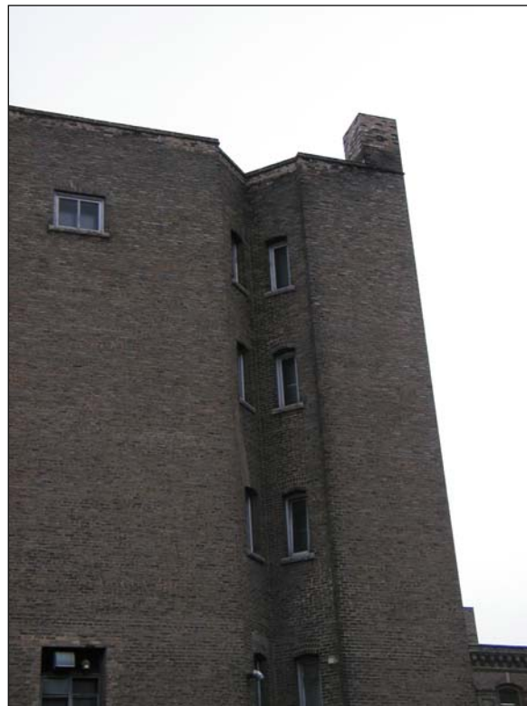
Plate 9 – Henderson Building, 332 Bannatyne Avenue, detail of west side window well. ( M. Peterson, 2005. )
