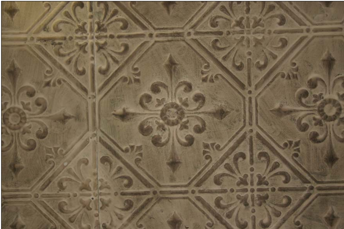
Plate 3 – Examples of the ornamental tin ceiling on the fourth floor (top) and in the basement (bottom). ( M. Peterson, 2005. )
