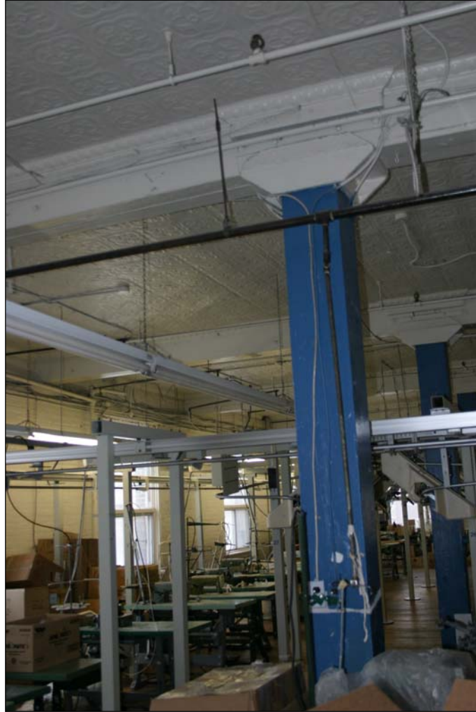
Plate 2 – Third floor, Henderson Building, 332 Bannatyne Avenue, example of the beam and post structural system. ( M. Peterson, 2005. )
