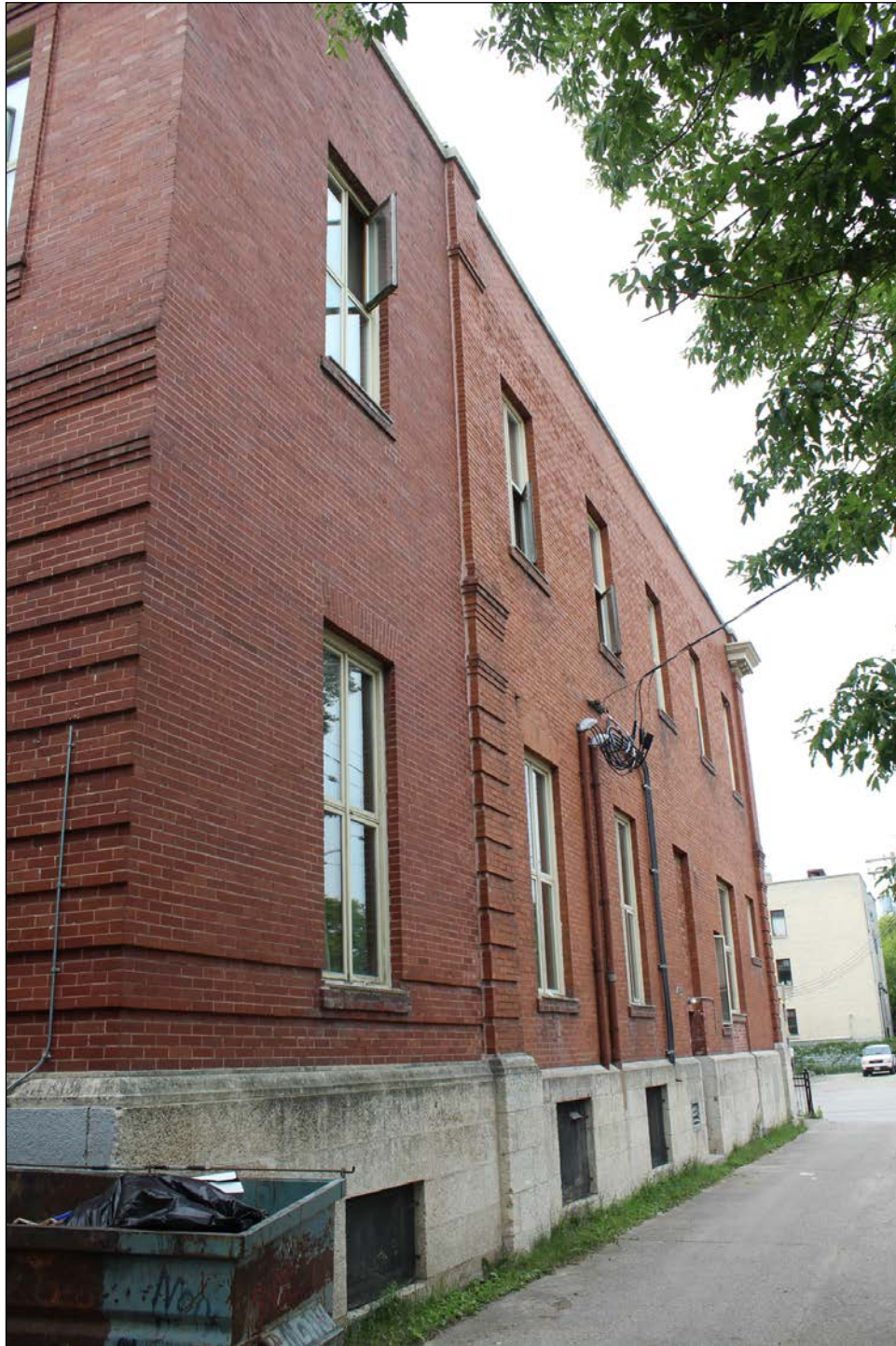
Plate 17 – Manitoba Telephone System – St. John's Exchange, 405 Burrows Avenue, rear (north) façade, 2017. (M. Peterson, 2017.)
