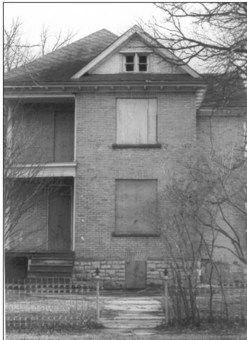
Plate 2 – Front (north) façade, which faces the Assiniboine River, no date. ( Courtesy of the City of Winnipeg, Planning Department. )
