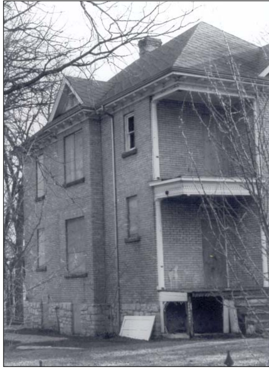
Plate 3 – Front (north) façade, with missing porch elements, no date. (Courtesy of the City of Winnipeg, Planning Department. )
