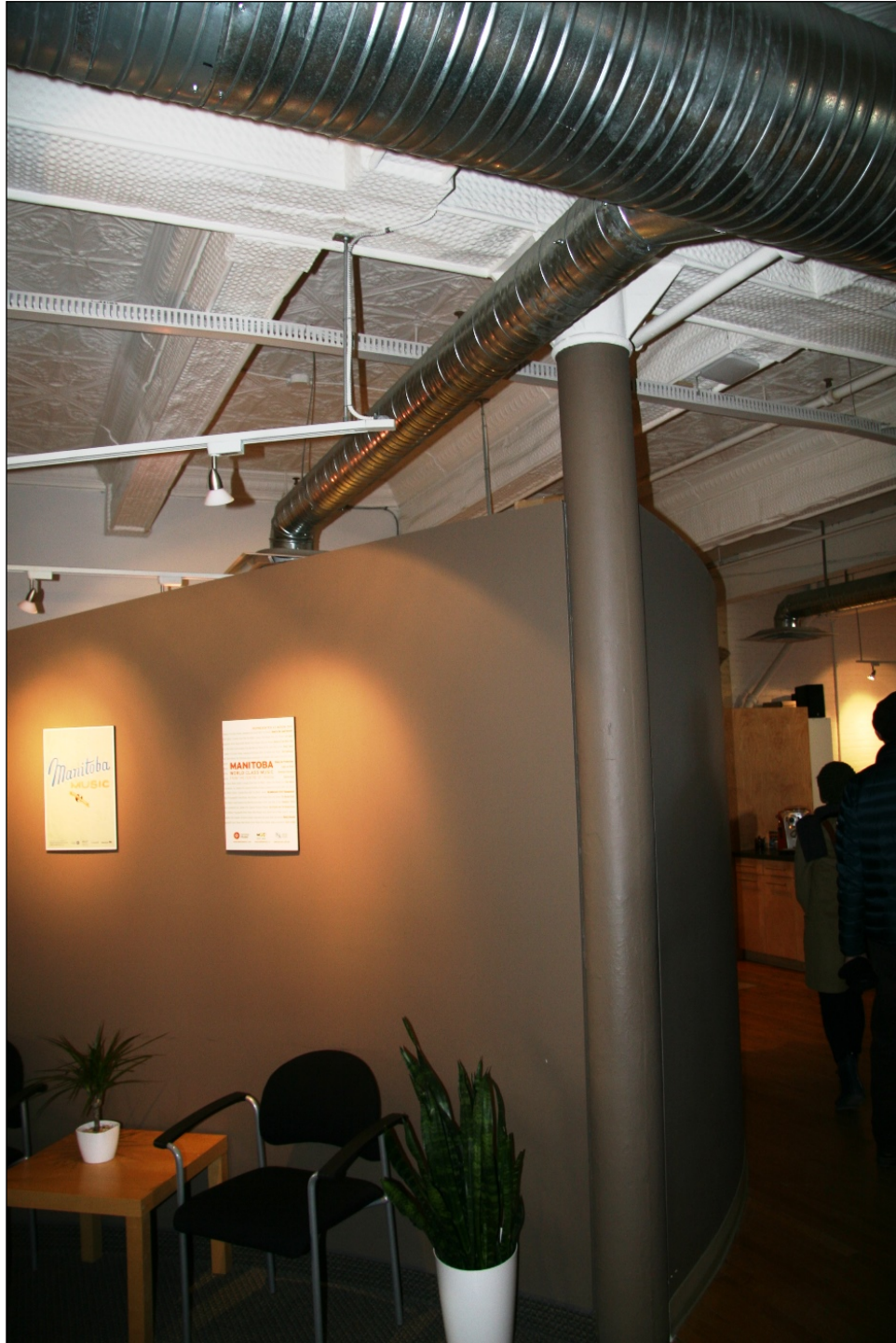
Plate 11 – Aldous Building, 376 Donald Street, cast iron post and ornamental tin ceiling, ground floor, 2015. (M. Peterson, 2015.)
