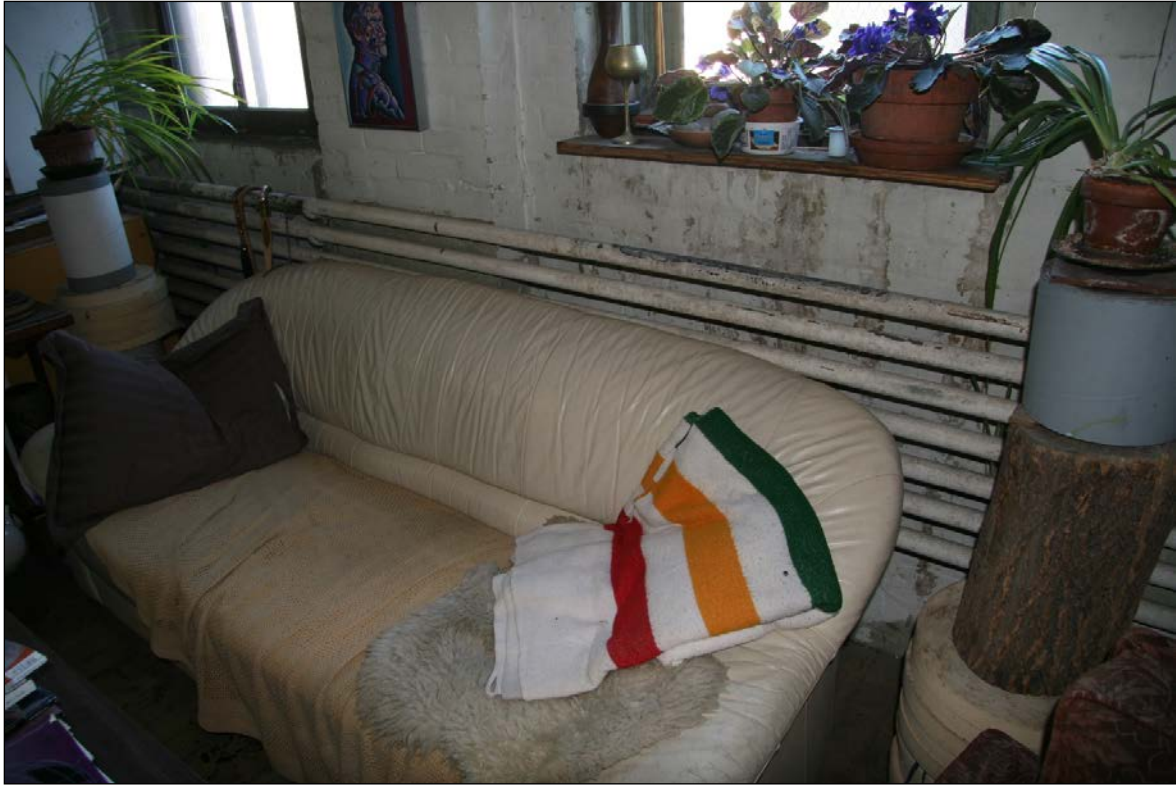
Plate 14 – Aldous Building, 376 Donald Street, 2 nd floor, original horizontal radiator piping, 2015. ( M. Peterson, 2015. )
