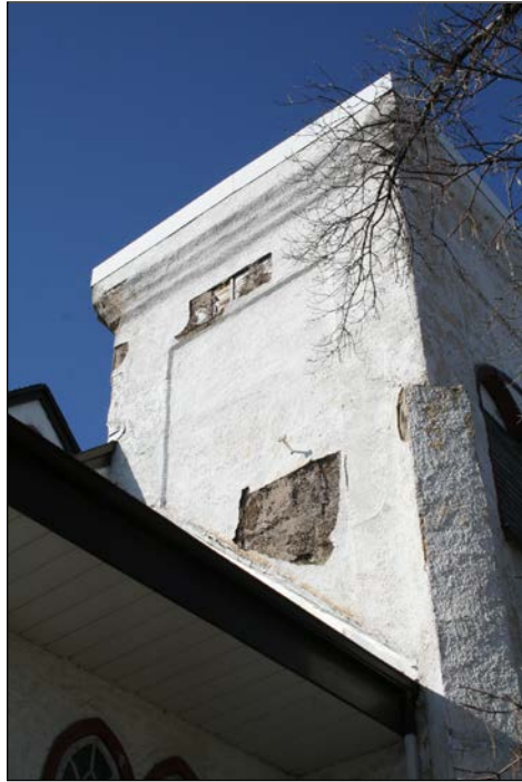
Detail of signs of aging on tower, 2009
