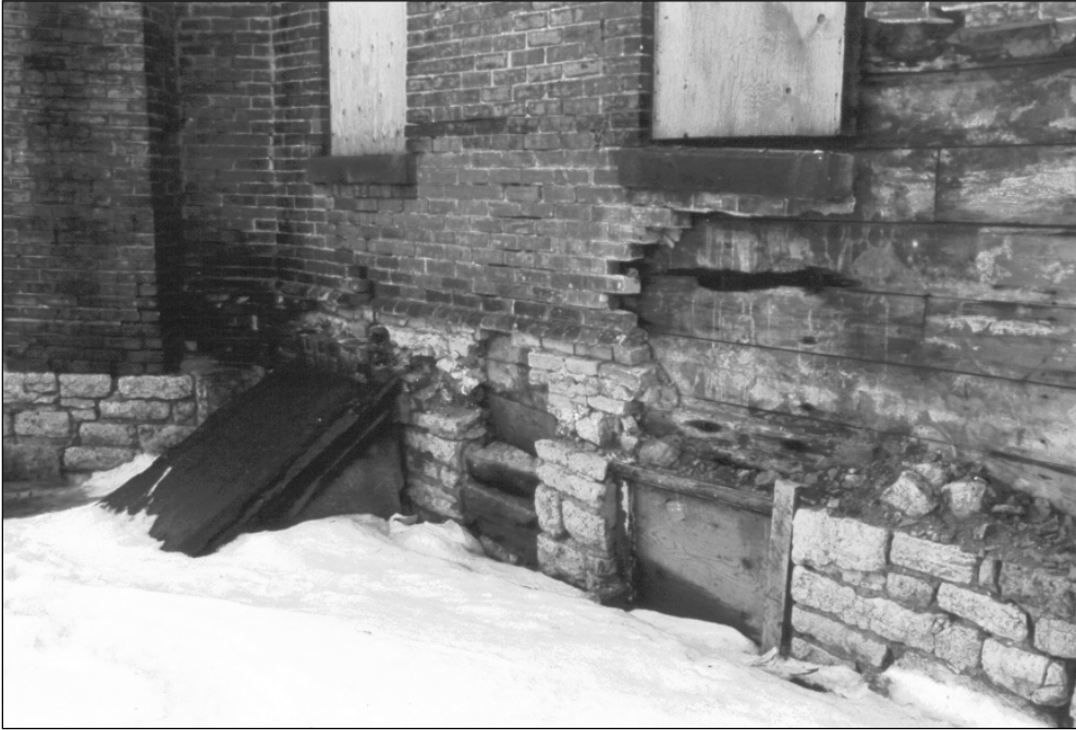
Plate 3 – Section of stone foundation and upper walls showing brick veneer loss and other signs of aging. (M. Peterson, 1987.)
