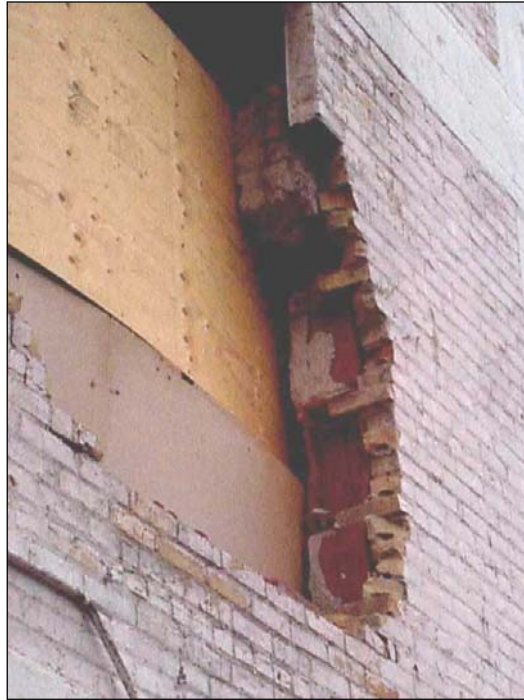
Plate 1 – New Hargrave Building, 361 Hargrave Street, detail of exterior wall construction, hollow tile and brick facing. ( M. Peterson, 2001. )
