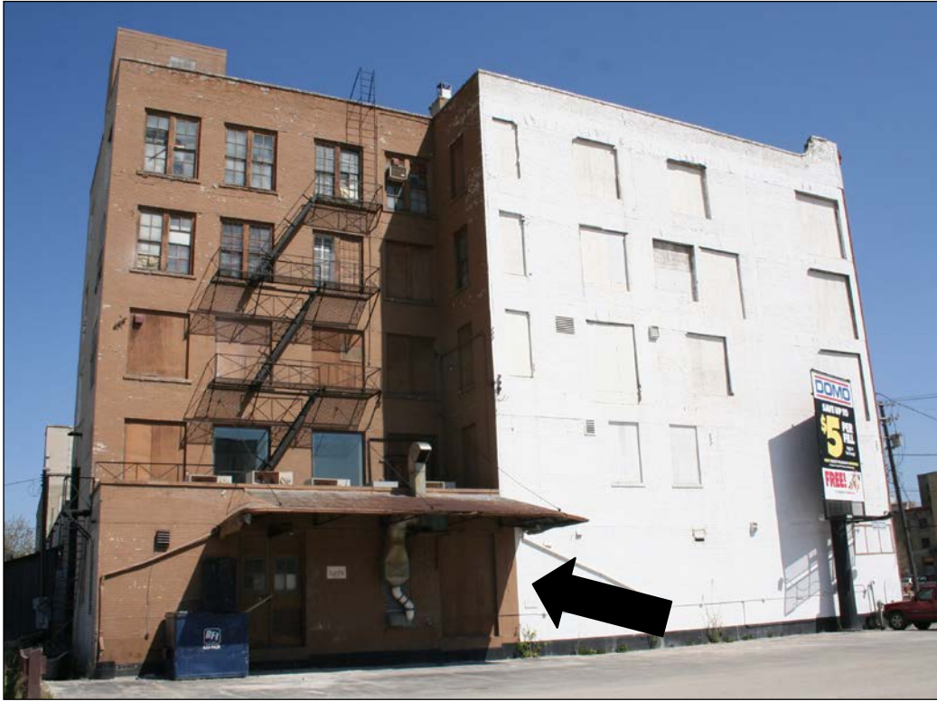
Plate 9 – Clark Brothers Warehouse, 448 Hargrave Street, south façade with 1952 loading area (arrow), 2006. (M. Peterson, 2006.)
