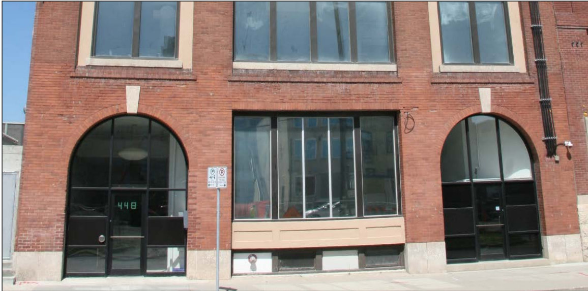
Plate 4 – Clark Brothers Warehouse, 448 Hargrave Street, detail of front (east) façade, 2015. (M. Peterson, 2015.)
