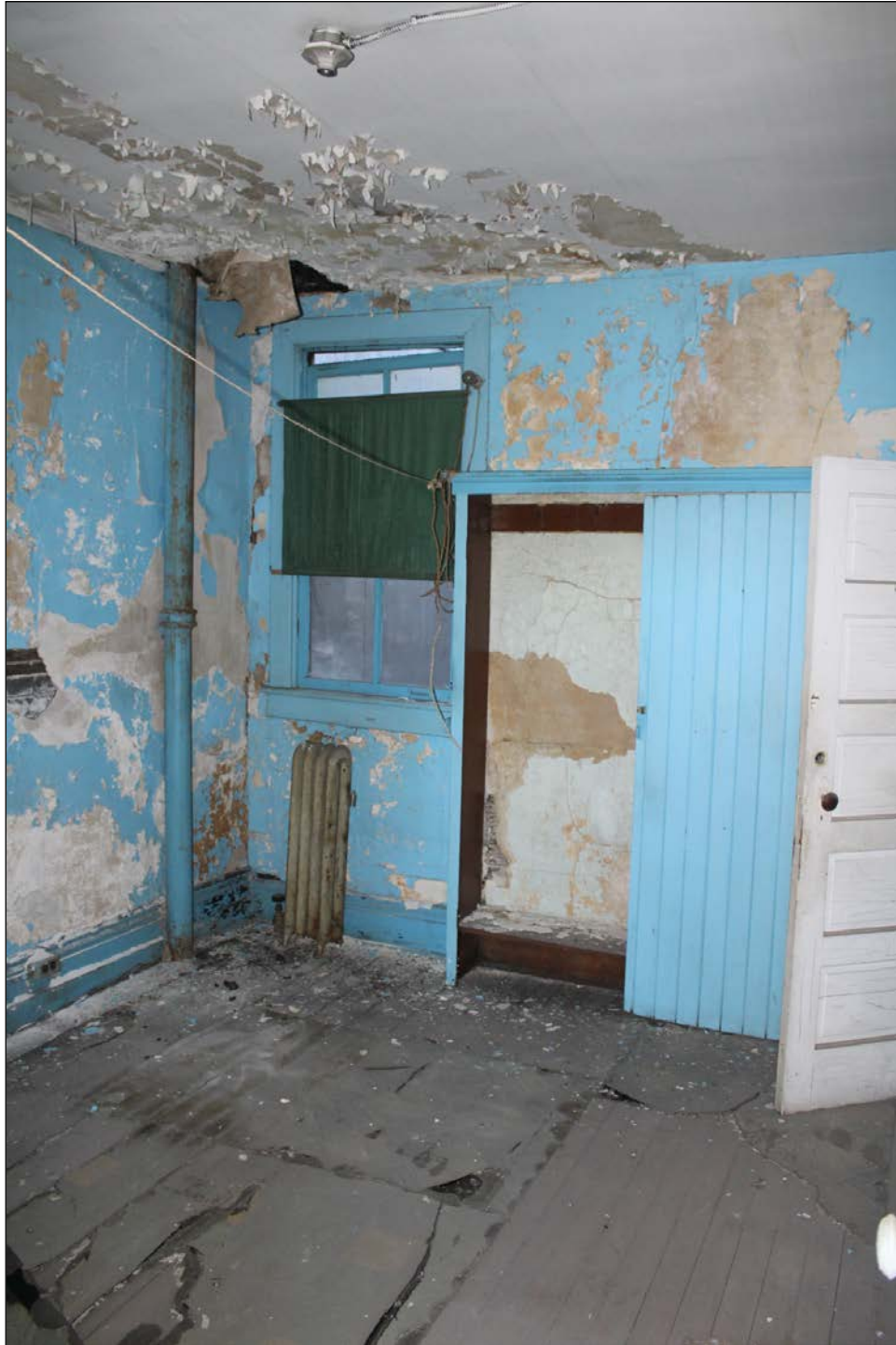
Plate 14 – Guest Block, 598 Main Street, deterioration in a third floor suite, 2015. ( M. Peterson, 2015. )
