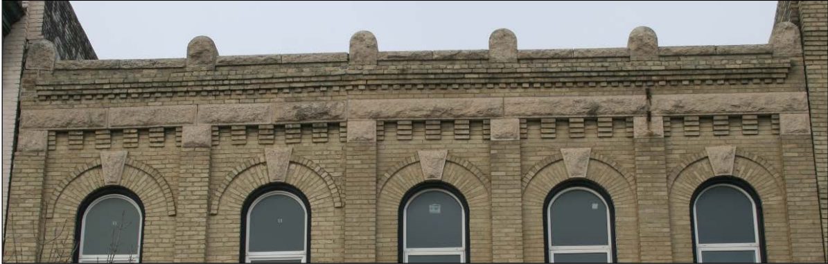
Plate 6 – Guest Block, 598 Main Street, front (east) façade, detail of roofline, 2014. (M. Peterson, 2014.)
