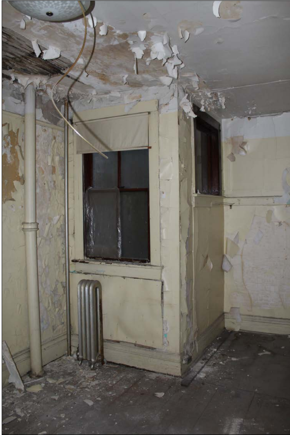
Plate 13 – Guest Block, 598 Main Street, deterioration in a second floor suite, 2015. ( M. Peterson, 2015. )
