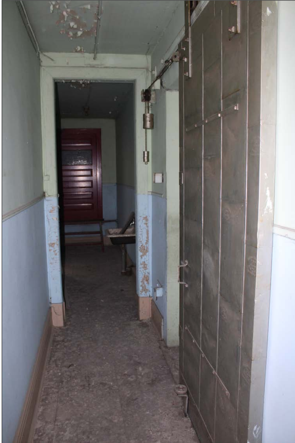
Plate 12 – Guest Block, 598 Main Street, fire door, third floor, 2015. ( M. Peterson, 2015. )
