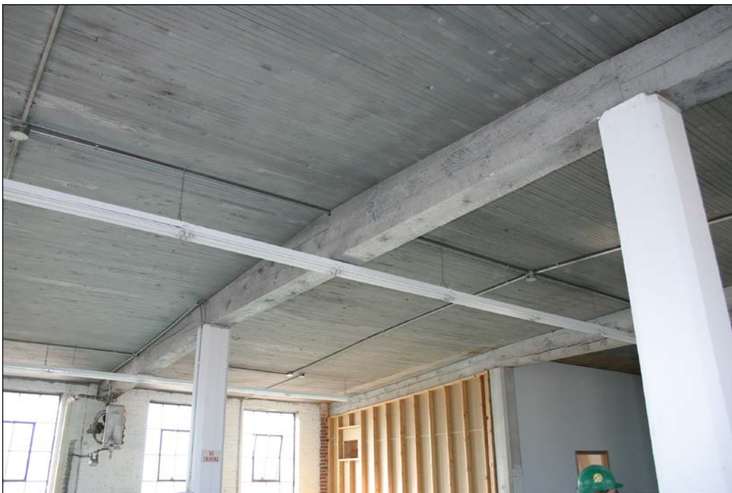
Plate 2 – 765 Main Street, Canadian Pacific Railway Post Office Building, third floor roof system, 2011. (M. Peterson, 2011.)
