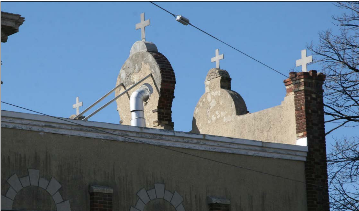
Plate 13 –Sts. Vladimir and Olga and Parish Hall, 115 McGregor Street, detail of front (west) façade, 2016. (M. Peterson, 2016.)
