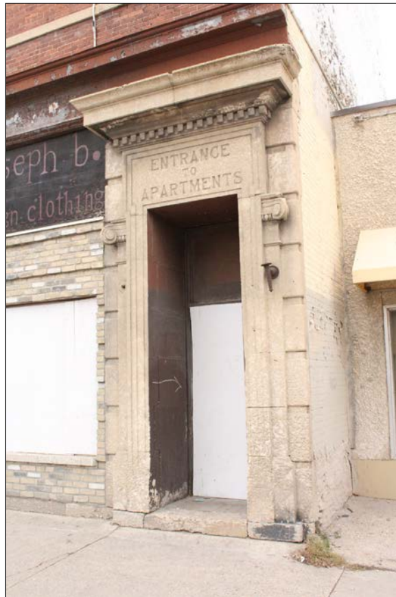
Plate 7 – Rubin Block/Morley Apartments, 270 Morley Avenue, details of north (top) and south (bottom) entrances, west façade, 2017. (M. Peterson, 2017.)
