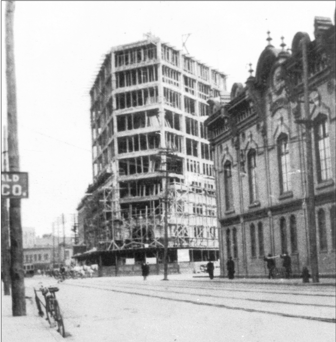
Plate 3 – The Lindsay Building during construction, Grace Methodist Church is on the right. ( Courtesy of the Provincial Archives of Manitoba. )
