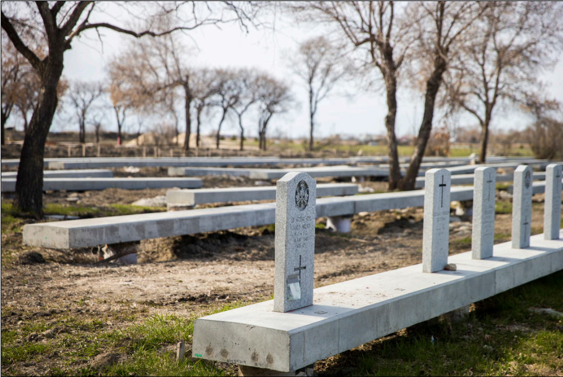
Plate 34 – Repairs and structural replacement in the Field of Honour, Brookside Cemetery, 2020. (Reproduced from Winnipeg Free Press, May 8, 2020, M. Mackenzie photographer.)
