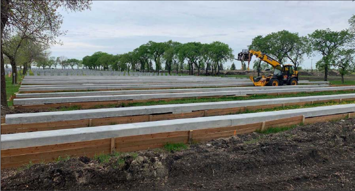
Plate 33 – Construction of new concrete beams in the Field of Honour, Brookside Cemetery by Manitoba company Haywood Concrete Products Limited, ca.2010. ( Reproduced from Haywood Concrete Products Ltd. website, https://haywoodconcrete.com/project-gallery . )
