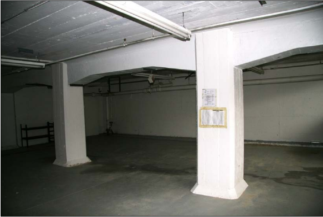
Plate 12 – Keewayden Block (Jacob-Crowley Building), 138 Portage Avenue, first floor concrete columns, 2016 (M. Peterson, 2016.)
