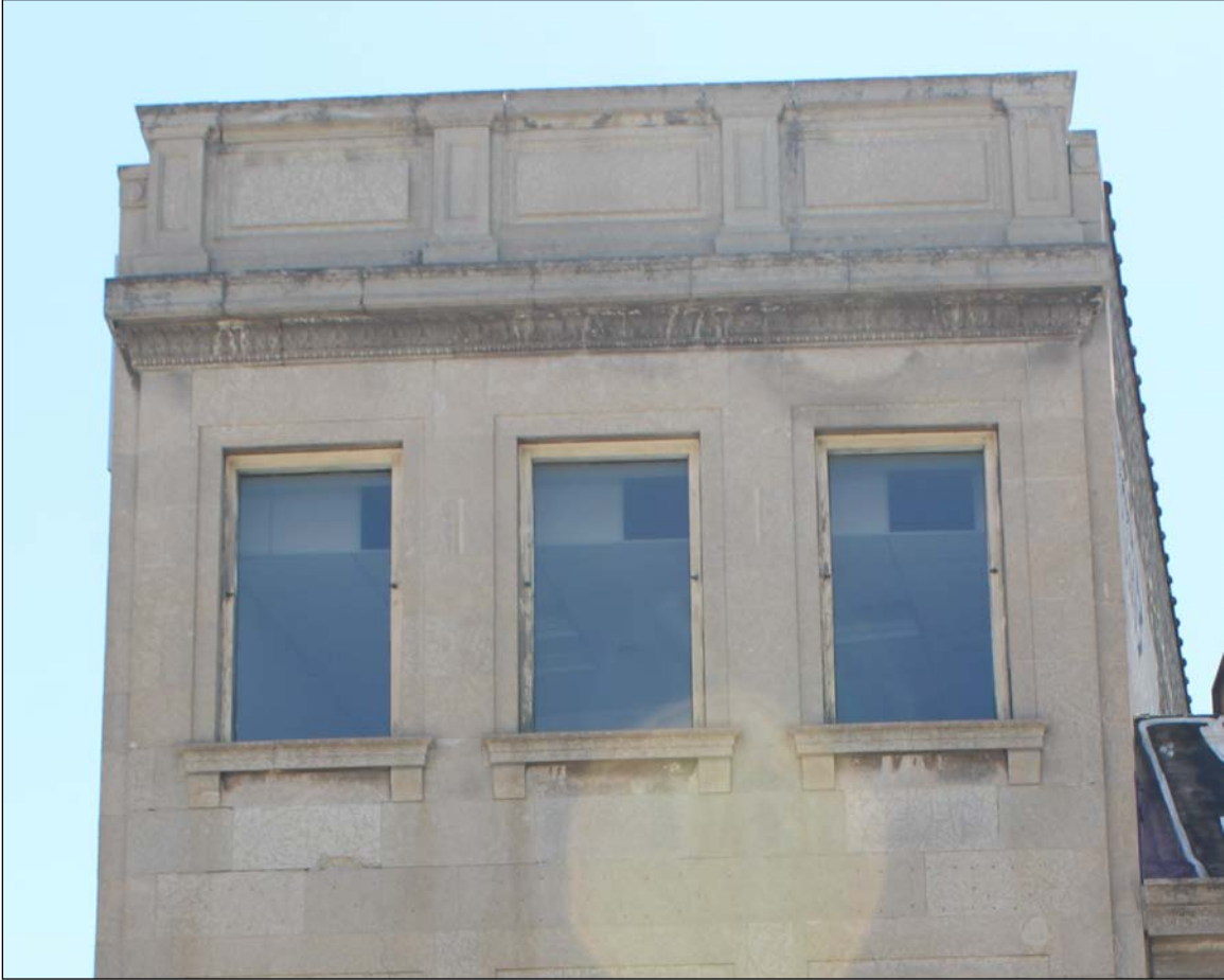
Plate 8 – Singer Sewing Machine Building, 424 Portage Avenue, detail of front (north) façade, 2019. ( M. Peterson, 2019. )
