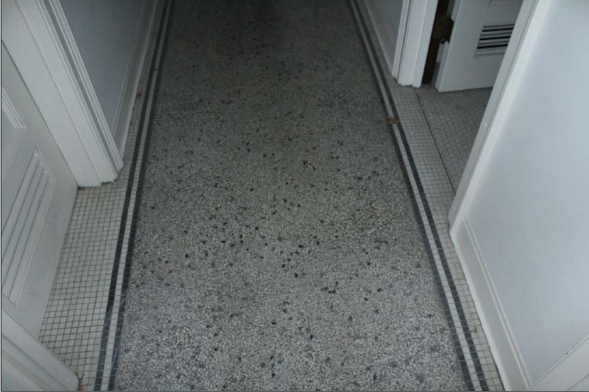
Plate 16 – Singer Sewing Machine Building, 424 Portage Avenue, second floor terrazzo and tile hallway flooring, 2019. (M. Peterson, 2019.)
