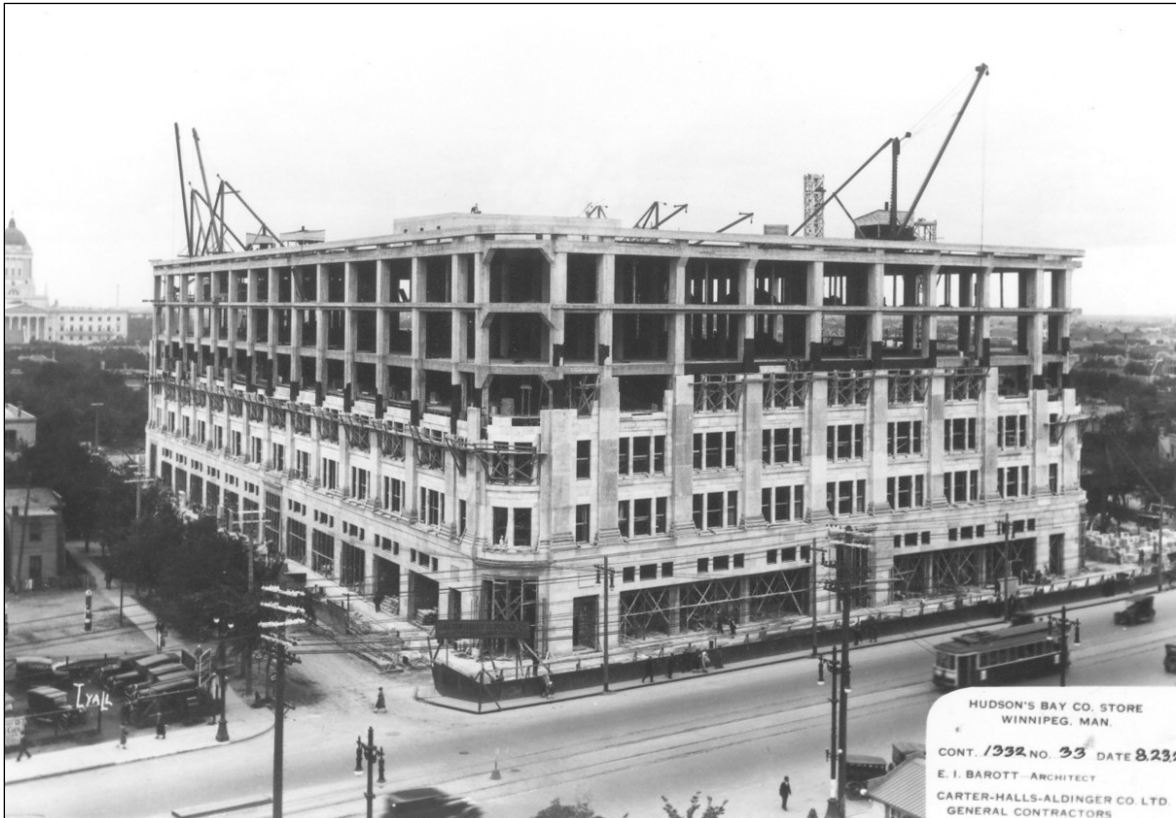
Plate 4 –Hudson’s Bay Company Store, 450 Portage Avenue, during construction, August 23, 1926. The parking lot that would become the Power Building is seen to the left. ( Hudson’s Bay Company Archives. )
