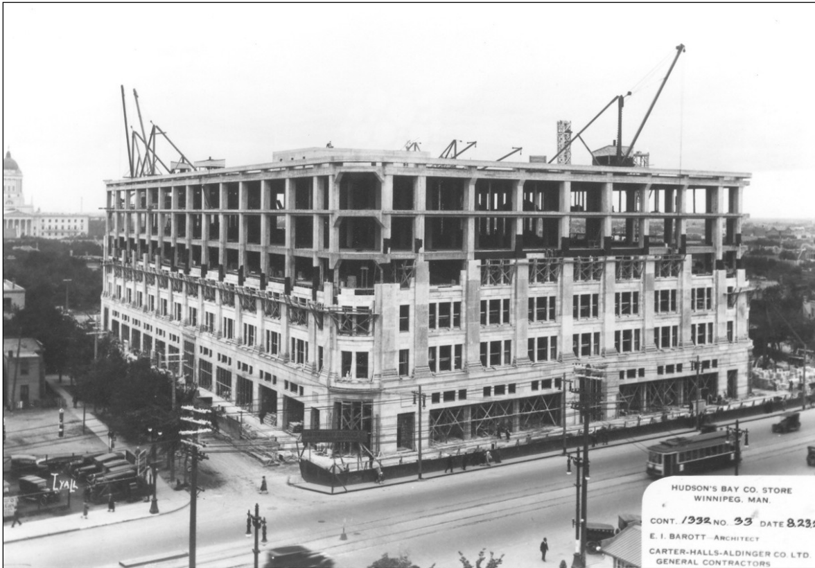
Plate 4 –Hudson’s Bay Company Store, 450 Portage Avenue, during construction, August 23, 1926. ( Hudson’s Bay Company Archives. )
