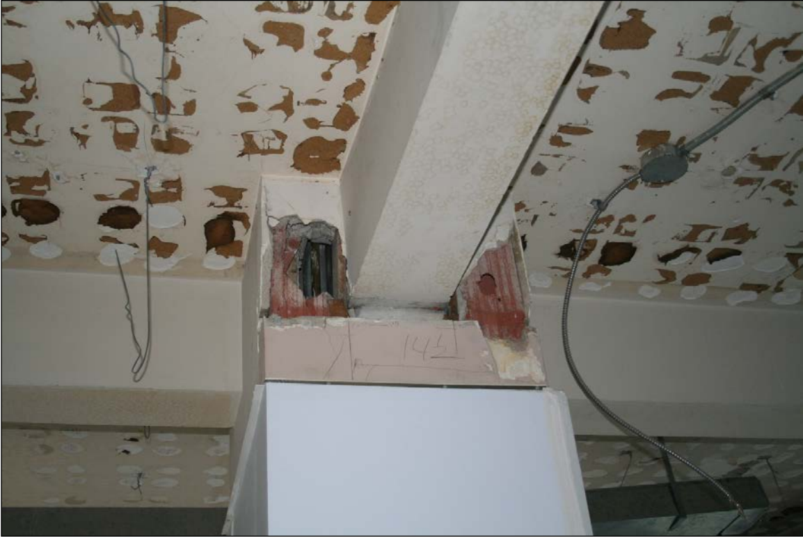
Plate 9 – Power Building, 428 Portage Avenue, example of reinforced concrete and hollow tile interior construction. (M. Peterson, 2006.)
