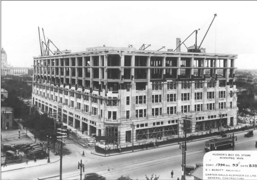
PLATE 27 - Construction of New Hudson’s Bay Company Store, 23 August 1926. The limestone sheathing of the first three floors has been completed in this view, and workers are beginning the fourth.
