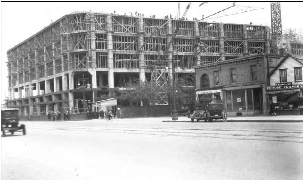
PLATE 25 - Construction of New Hudson's Bay Company Store, Looking Southeast from Portage Avenue and Balmoral Street, May 1926. The huge size of the uncompleted department store, as well as its heavy reinforced concrete skeleton are quite apparent in this view. ( Manitoba Archives )
