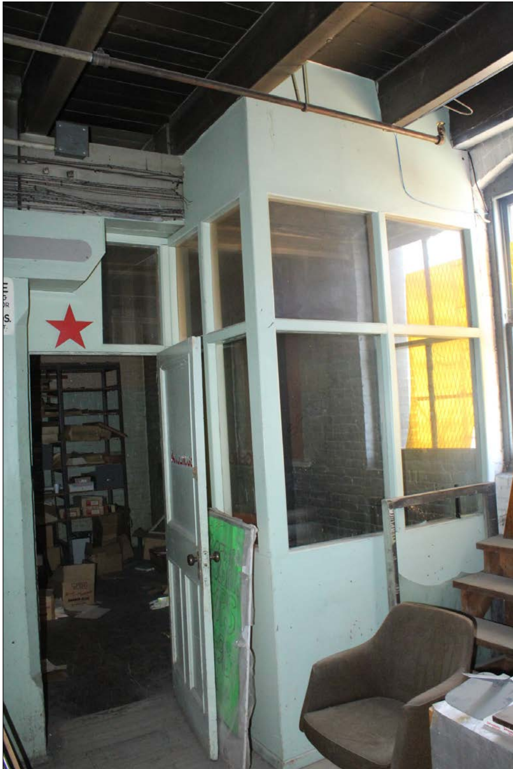
Plate 19 – Cockshutt Plow Company Building, 238 Princess Street, second floor office partitioning, 2019. (M. Peterson, 2019.)
