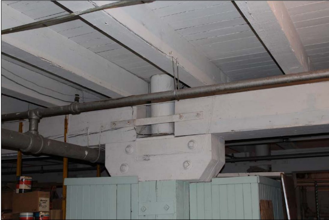
Plate 14 – Cockshutt Plow Company Building, 238 Princess Street, basement beam and post construction, 2019. (M. Peterson, 2019.)
