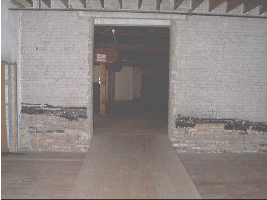
Plate 7 – Fourth floor interior doorway leading from former 78-84 to 86-88 Princess Street. ( M. Peterson, 1998. )
