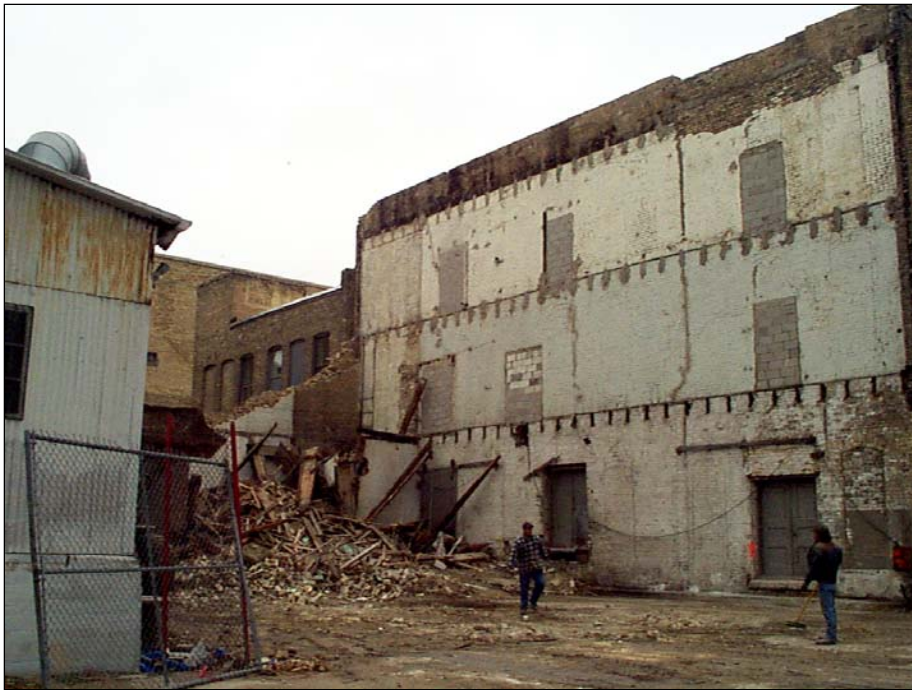
Plate 4 – Demolition of the rear addition of the Bathgate Block, October 2000. (M. Peterson, 2000.)
