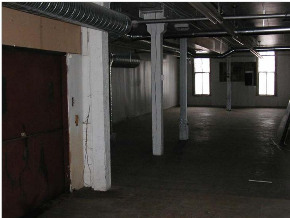
Plate 12 – Second floor posts, original wooden elements in foreground, steel replacement posts to rear (east end), 2004. (M. Peterson, 2004.)
