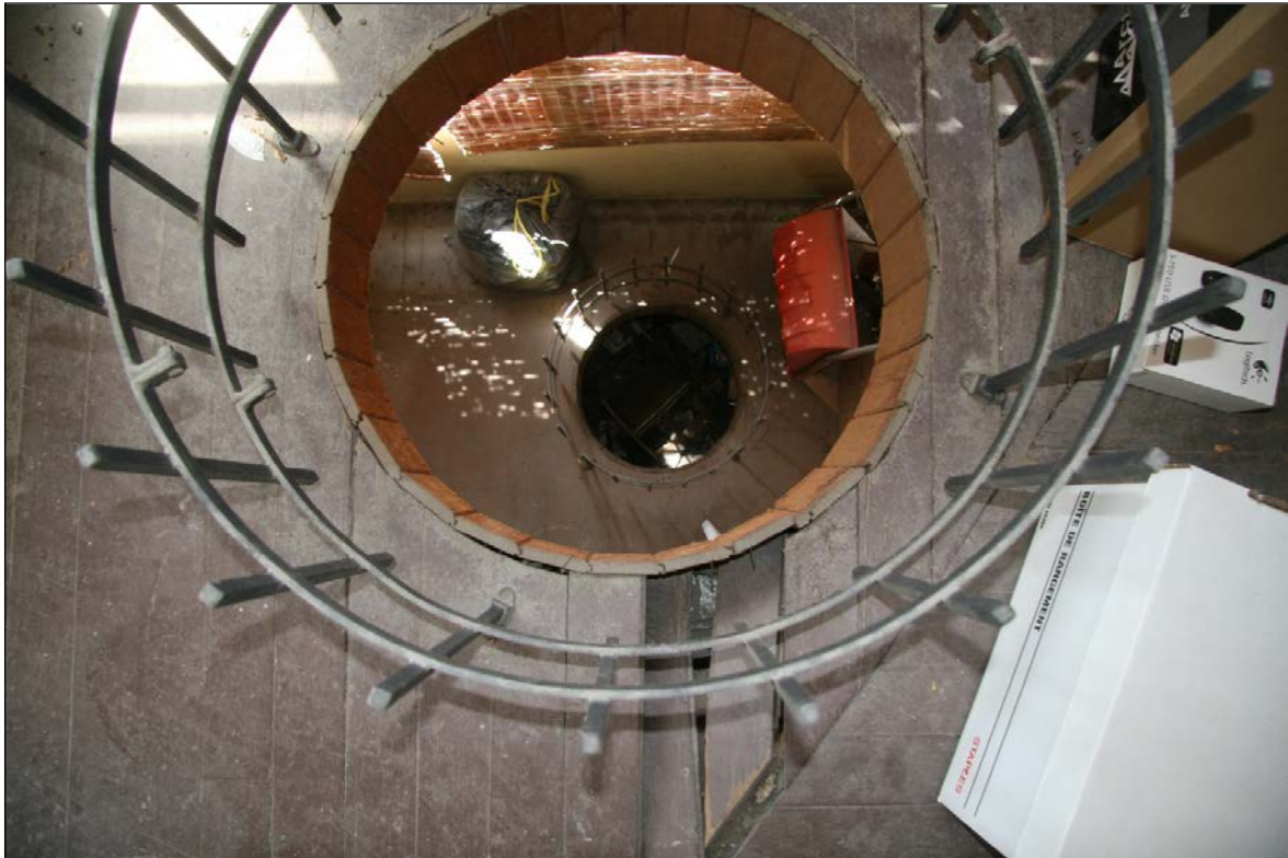
Plate 18 – Leslie Ironside House, 94 Roslyn Road, porch looking down from the second floor, 2018. ( M. Peterson, 2018. )
