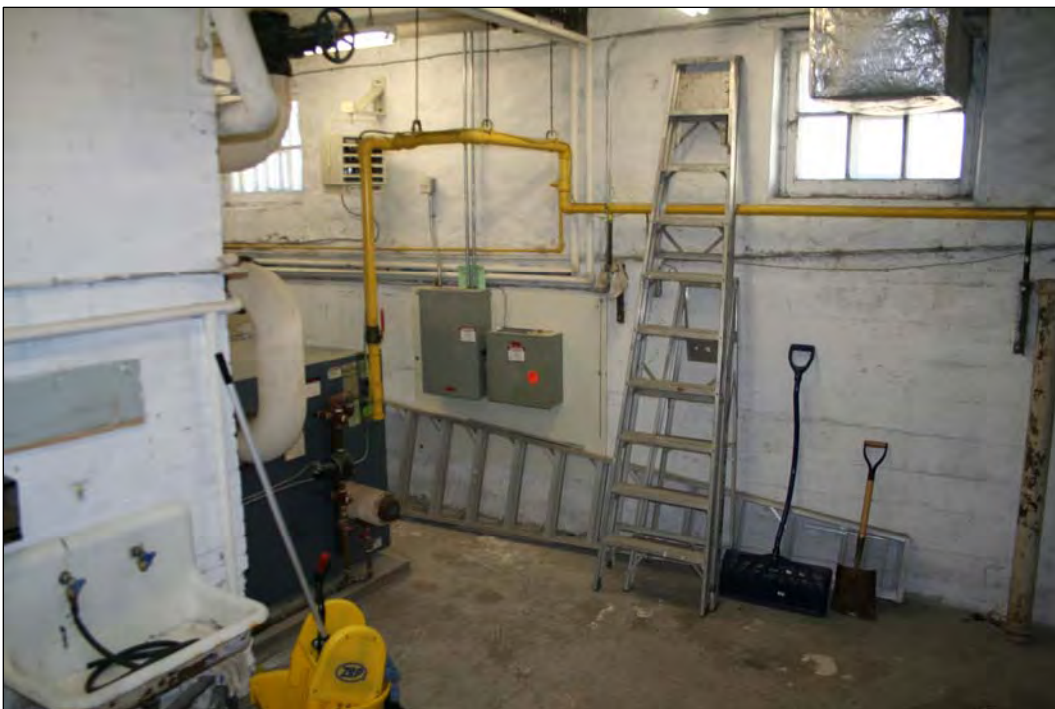
Plate 18 – St. John’s Library, 500 Salter Street, basement boiler room, 2010. ( M. Peterson, 2010. )
