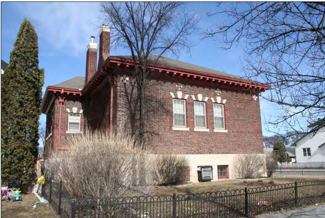
Plate 13 – St. John’s Library, 500 Salter Street, rear (west) and south façades, 2010. ( M. Peterson, 2010. )
