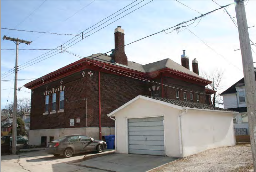
Plate 12 – St. John’s Library, 500 Salter Street, rear (west) and north façades, 2010. ( M. Peterson, 2010. )
