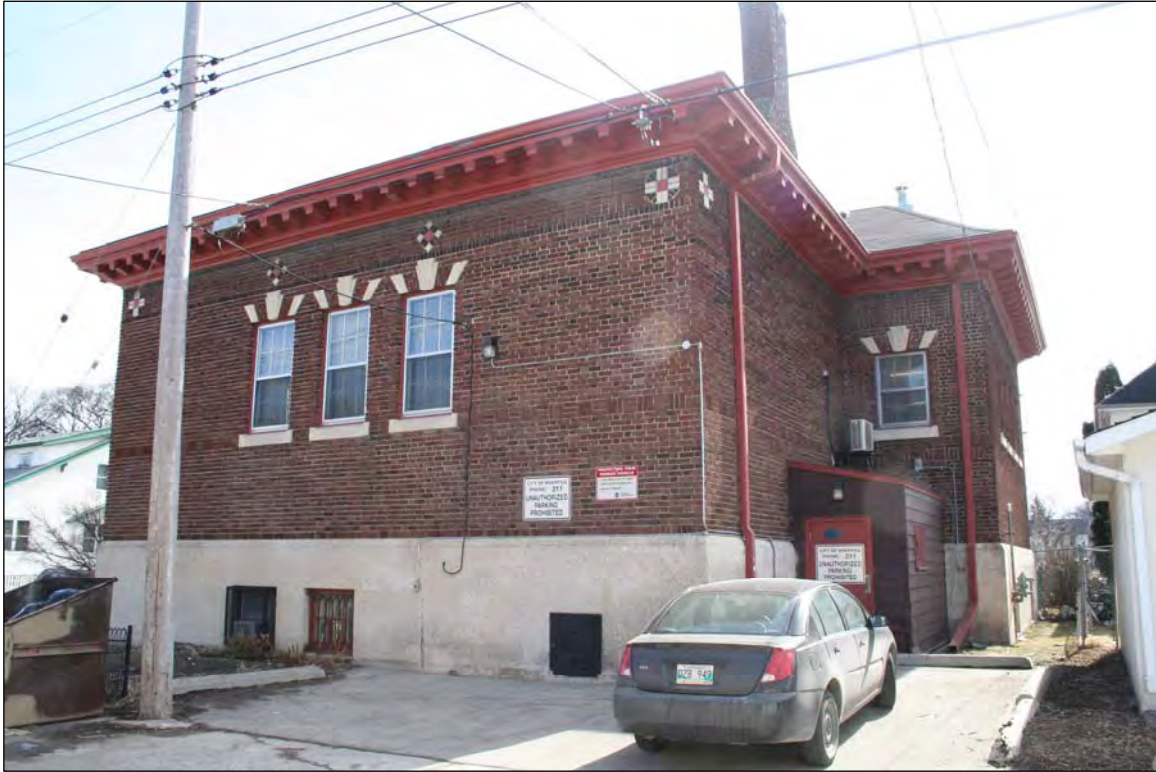
Plate 11 – St. John’s Library, 500 Salter Street, rear (west) and north façades, 2010. ( M. Peterson, 2010. )
