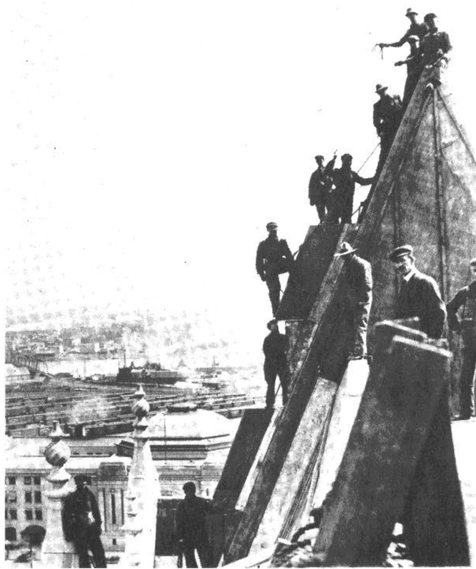
Workers sheathing the roof of the Fort Garry Hotel in copper, circa 1913.
