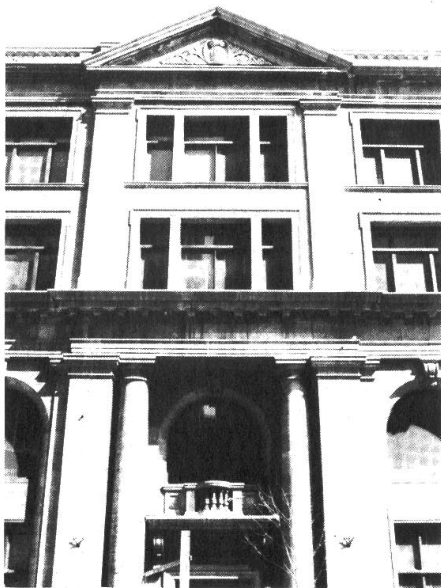
The Victory Building's Bedford stone facade, illustrating ornamental balcony at second floor.
