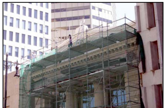
Workmen repairing the magnificent terra cotta on the Oldfield Kirby Gardner Building, 234 Portage Avenue
