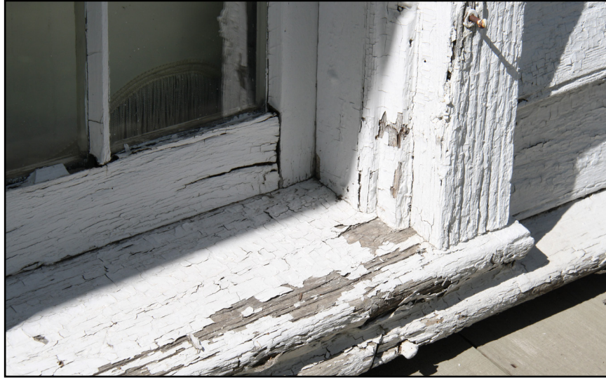
115 Rupertsland Boulevard, deteriorated wood windowsill
