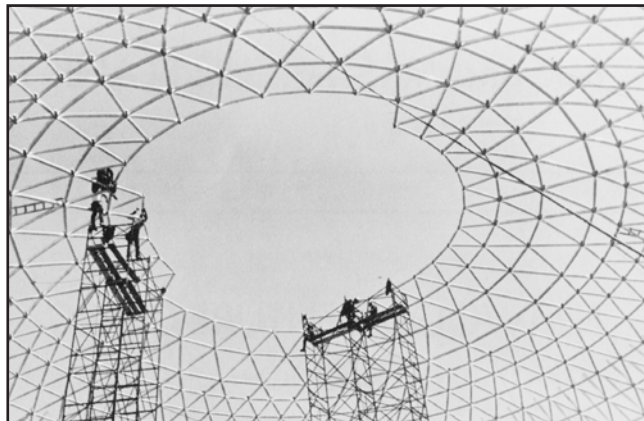
Rainbow Stage, 2015 Main Street, Kildonan Park, 1970 construction of the domed roof. (J. Olenko image)
